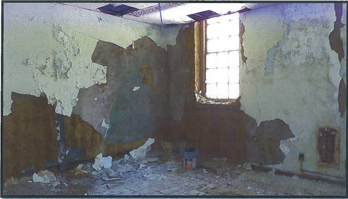
Condition of the wire mesh that supported the plaster on the second floor. Behind this, the salmon brick is saturated. Many bricks are crumbling from freeze-thaw cycles and must be replaced, or the wall rebuilt.
