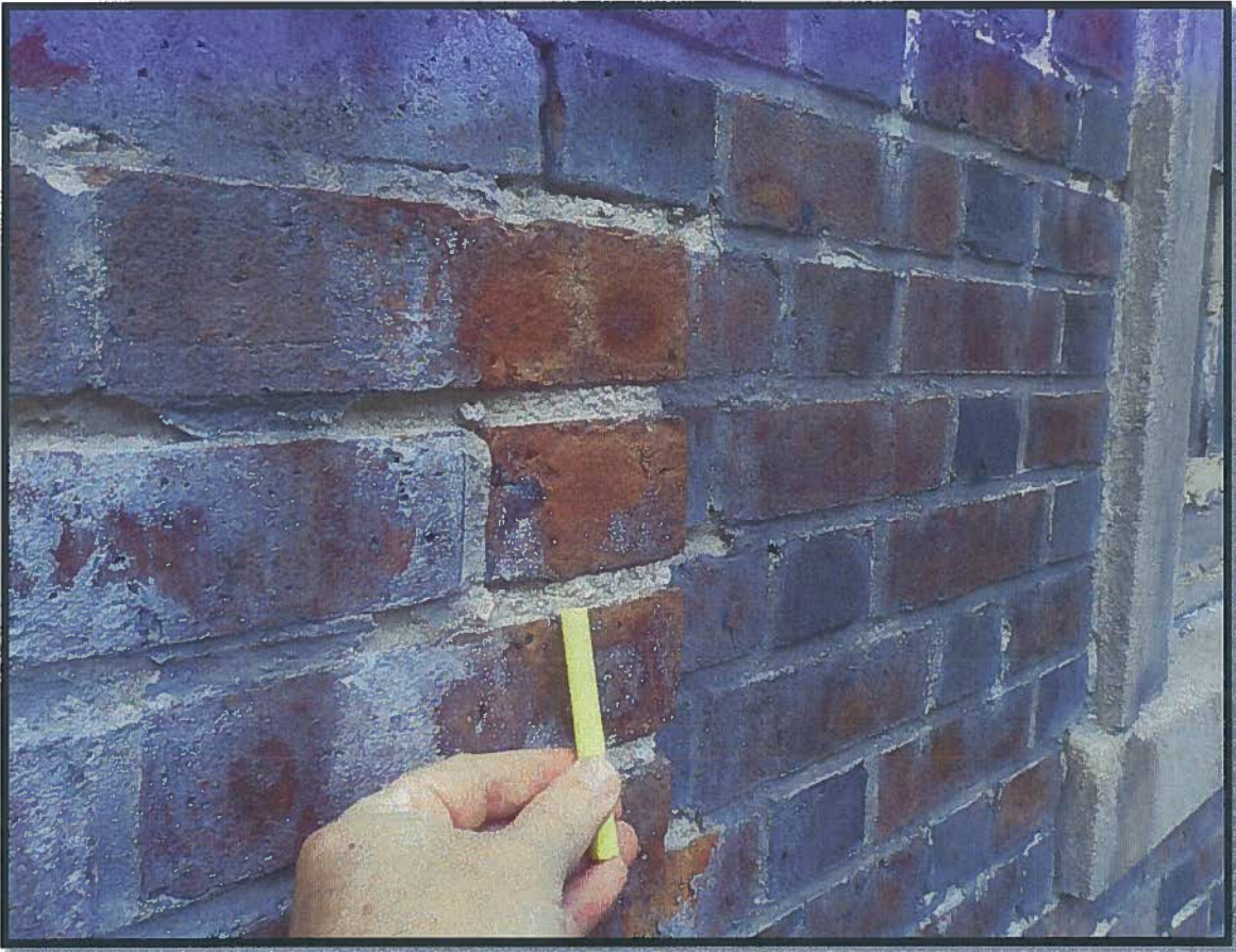
The water migration has washed out the calcium and caused the mortar to turn to powder due to freeze-thaw cycles.
