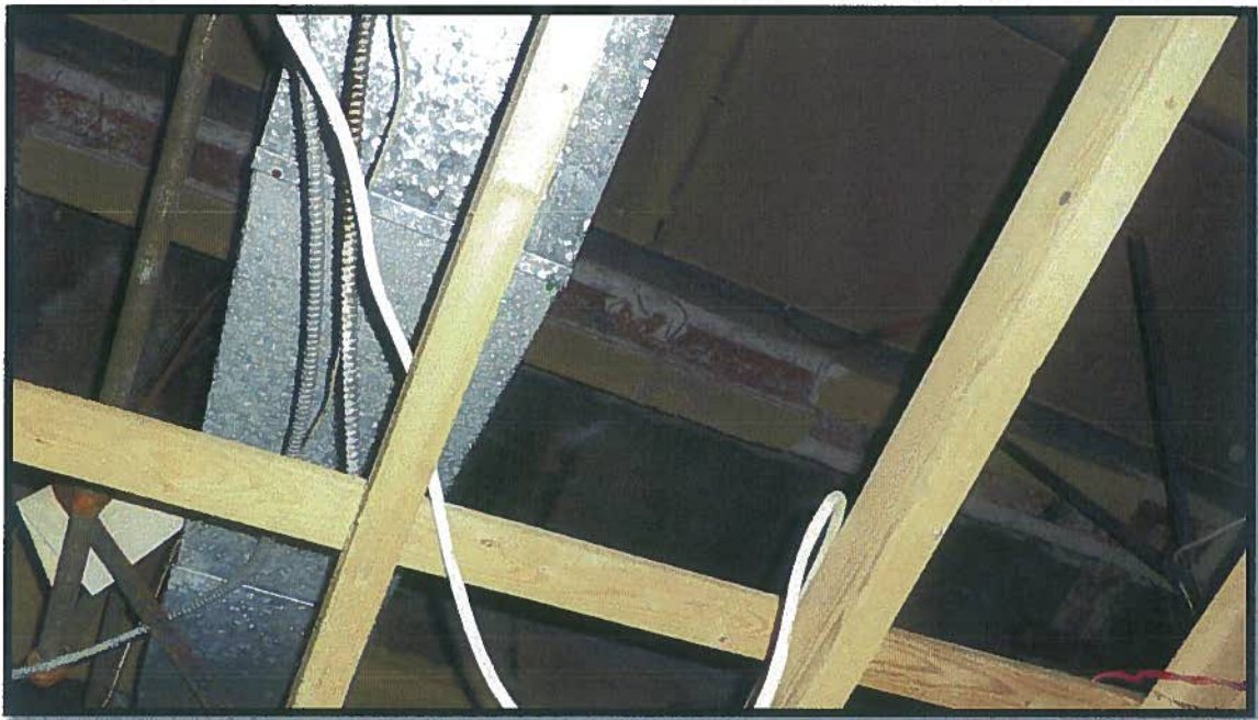
Concrete encasement is spalled at the underside of the beam due to corrosion (rust jacking).
