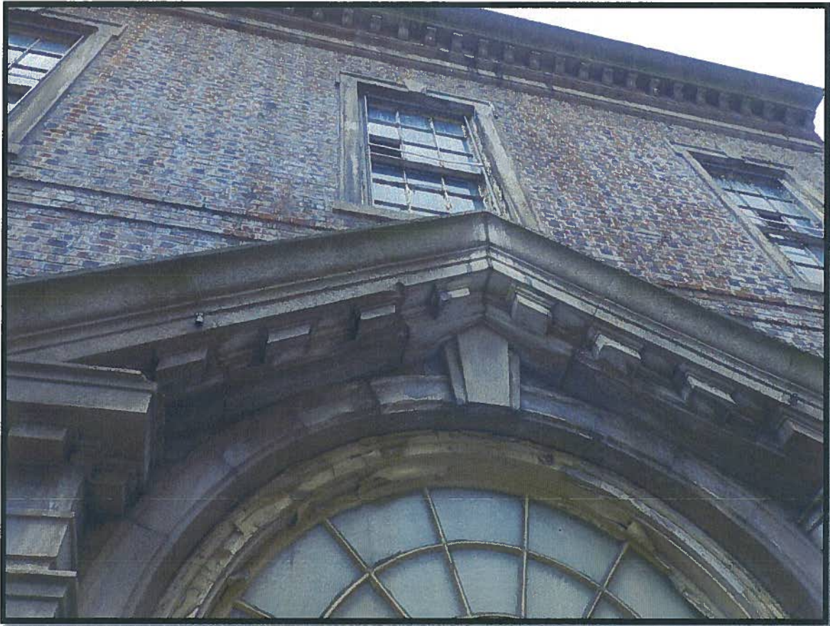
A tremendous volume of water permeation over many years left extensive salt deposits and damaged embedded wood elements such as window frames.
