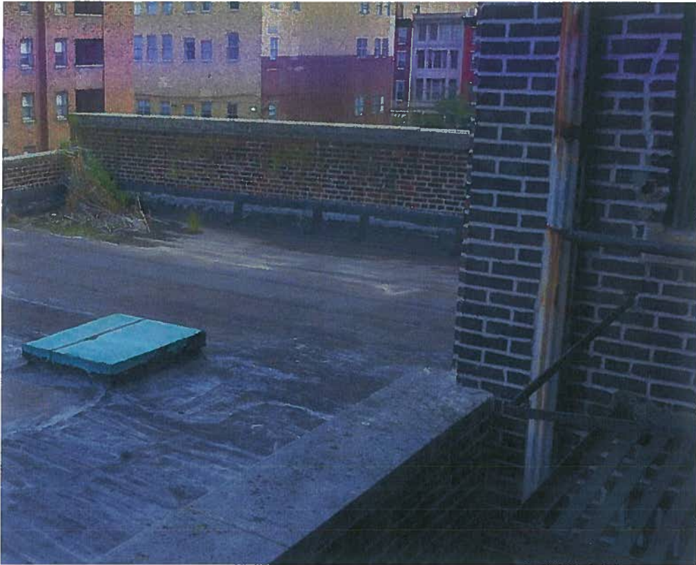
1918-1920 Sansom Street, levels of water damage in parapet and roof from blocked drains (August 2015)
