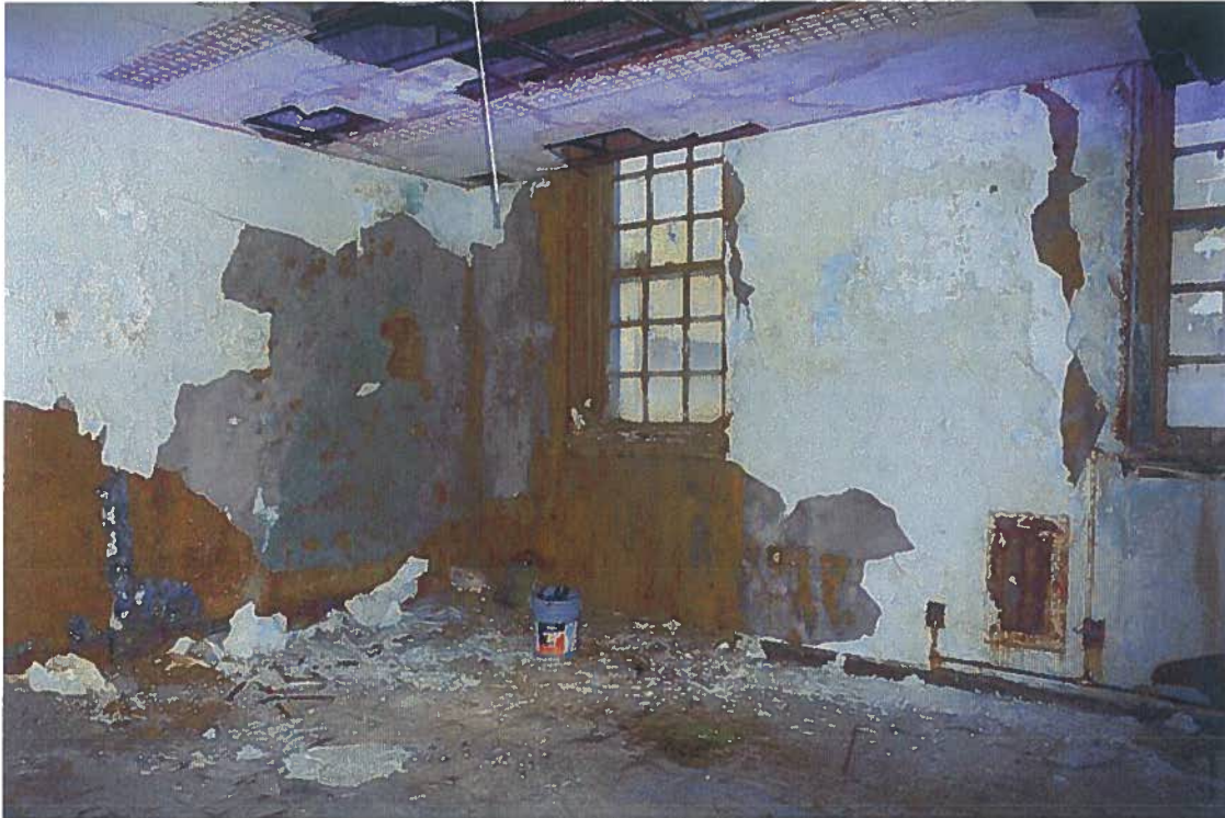
1918-1920 Sansom Street, NW corner second floor front, multiple layers of wire lath and plaster, destroyed by water; suspended ceiling (August 2015)
