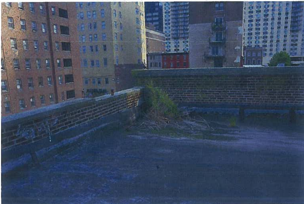
1918-20 Sansom Street, plants growing in roof drains, evidence of level of roof water damage
