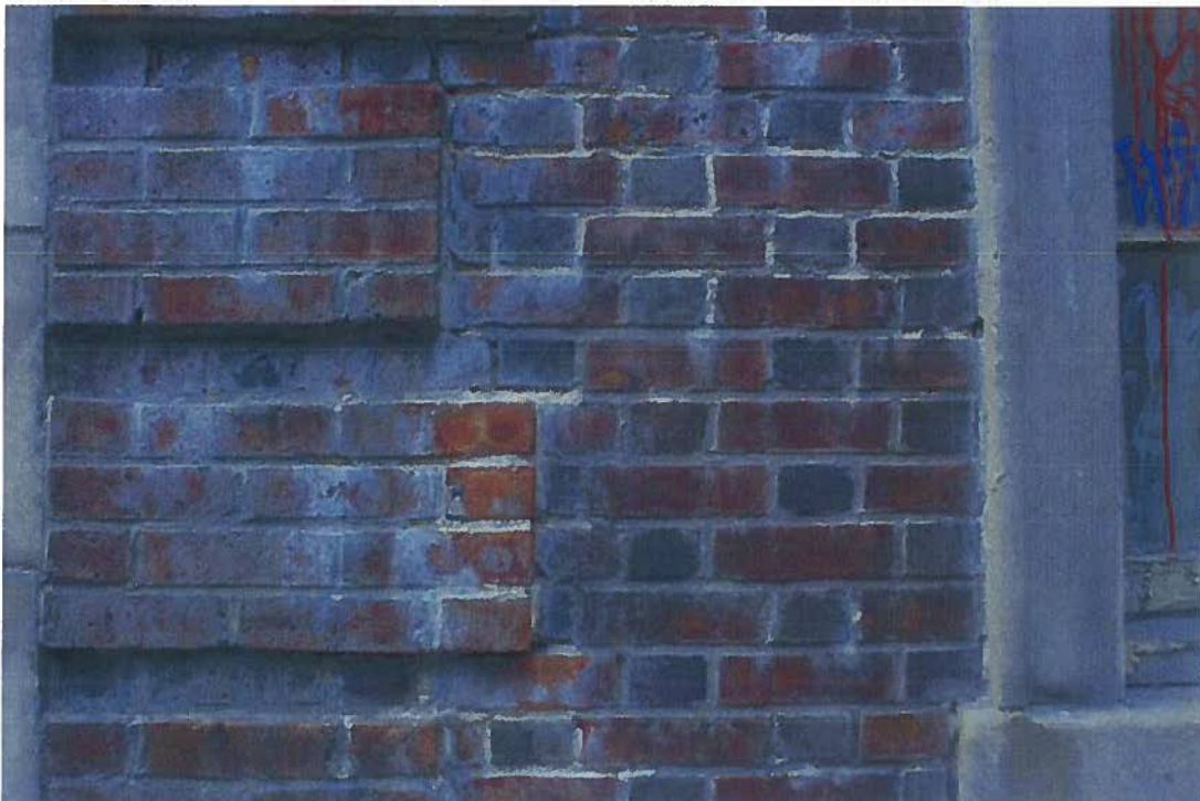
1918-20 Sansom Street, water staining, spalling and efflorescence through brick and stone, Sansom Street façade (August 2015)
