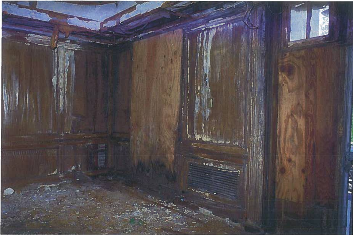
1918-20 Sansom Street, front lobby, NW corner, showing extent of water damage from roof drains (August 2015)
