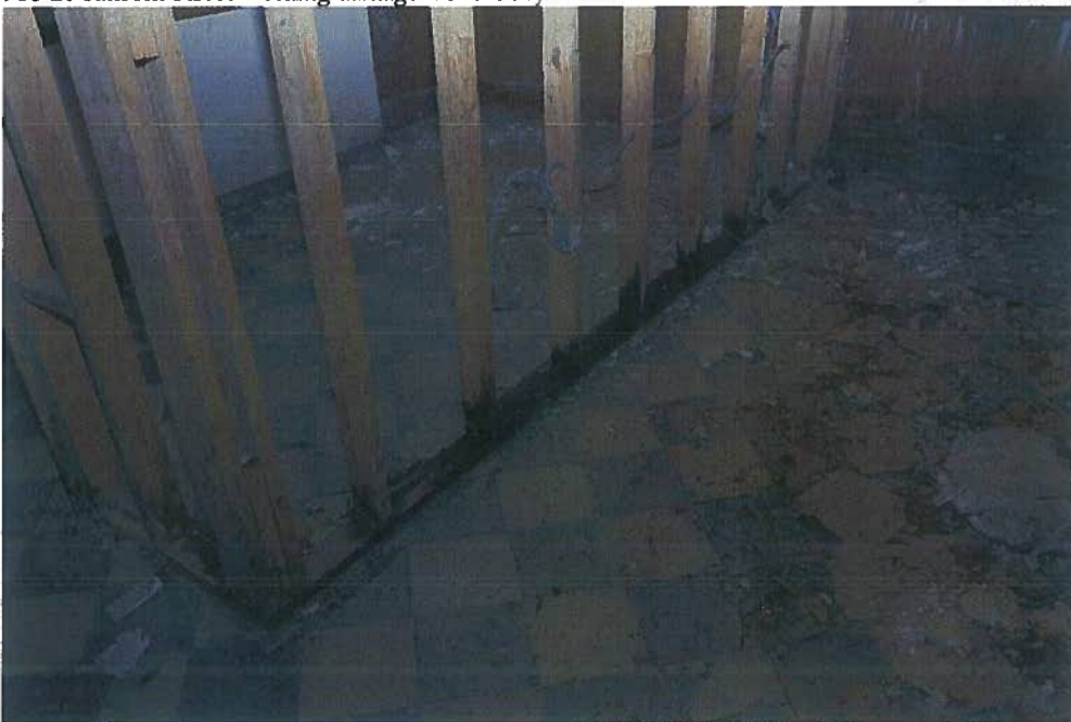
1 1918-20 Sansom Street, rot damage to modern partition (August 2015)
