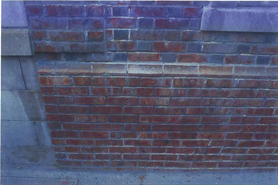
1918 -20 Sansom Street, water staining, spalling damage, and overpointing, brick of Sansom Street façade (August 2015)
