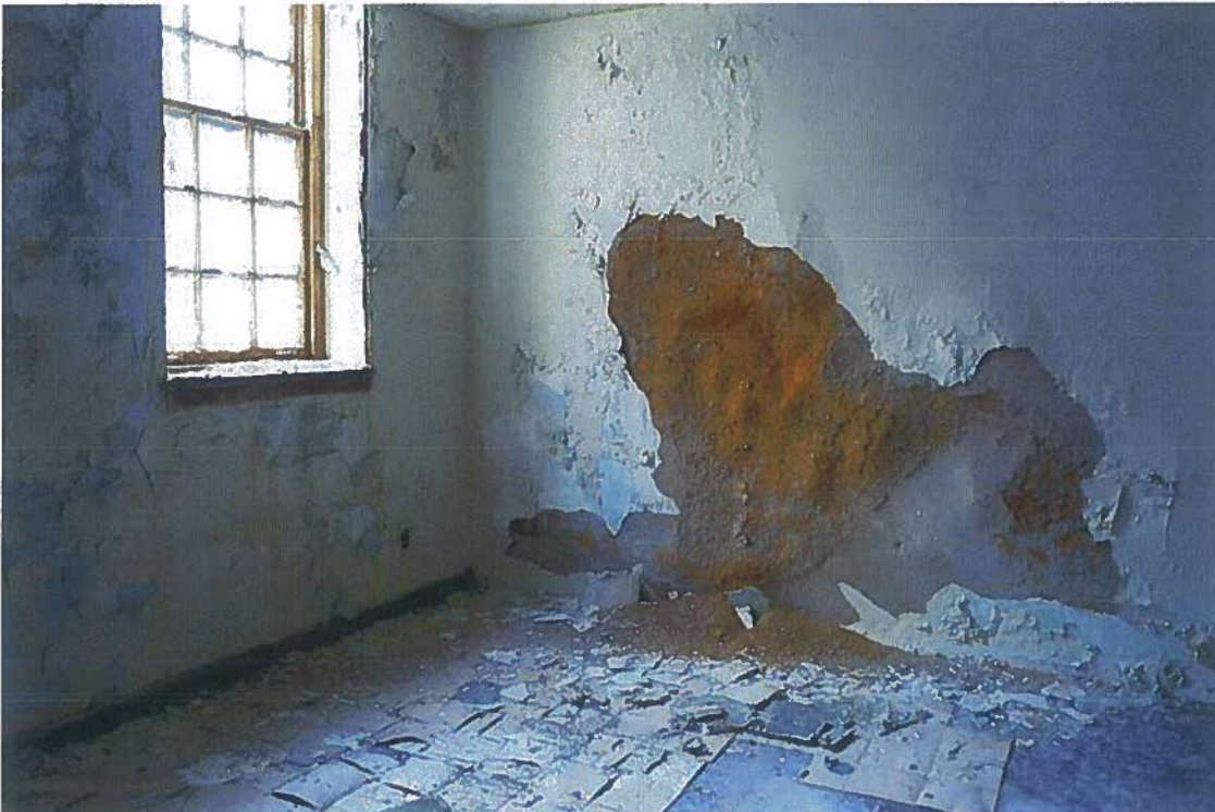
1918-20 Sansom Street, NE corner, second floor front, destroyed wire lath, east wall under failed roof drain (August 2015)
