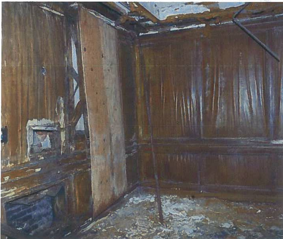
1918 -20 Sansom Street, front lobby NE corner, showing extent of water damage from roof drains, (August 2015)
