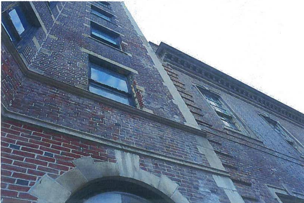
1906-12 and 1918-1920 Sansom Street, efflorescence and water damage where 1918 -1920 roof drains cause leakage into both buildings
