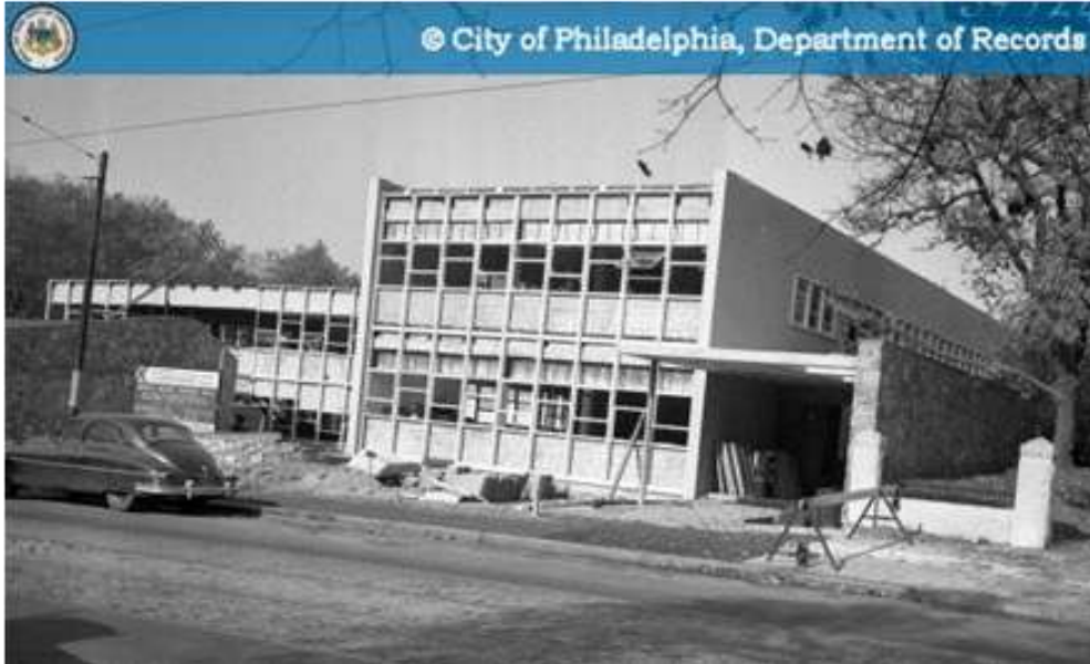
Figure 14A: District Health Center 3, 4217 Chester Ave., under construction, November 10, 1959 (PhillyHistory.org, Philadelphia Department of Records)
