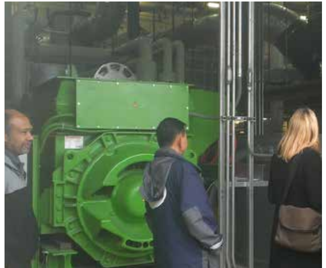
Visitors take a look at one of the four cogen engines.
