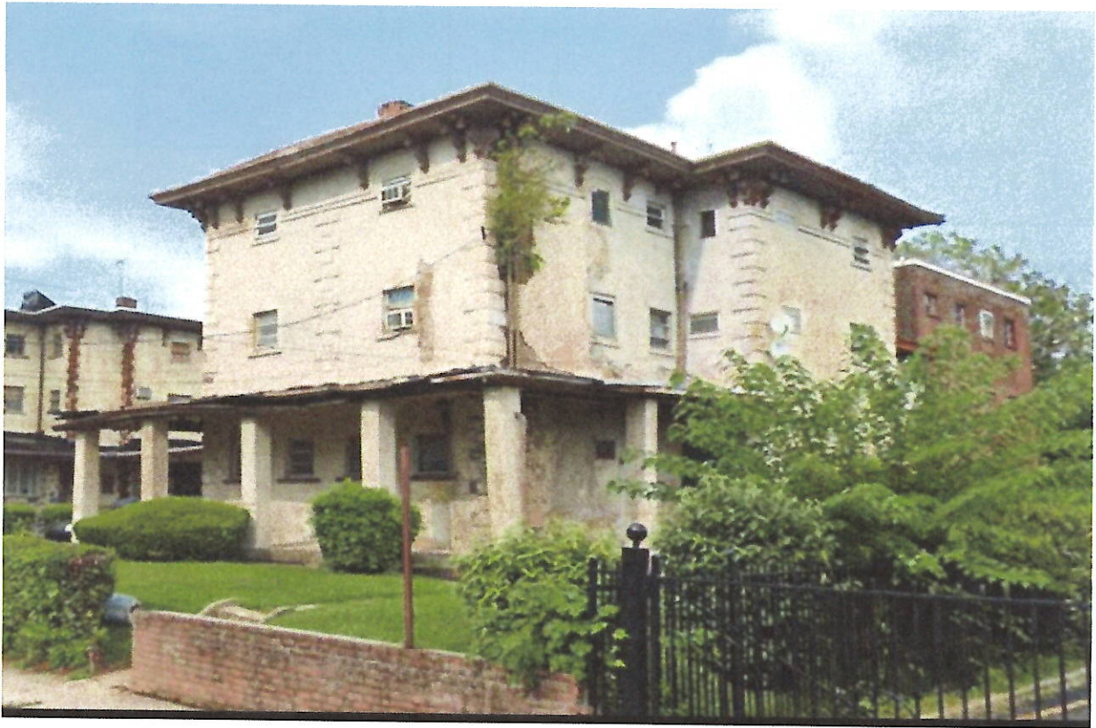
Photo # 3: showing structural damages to the porch roof.
