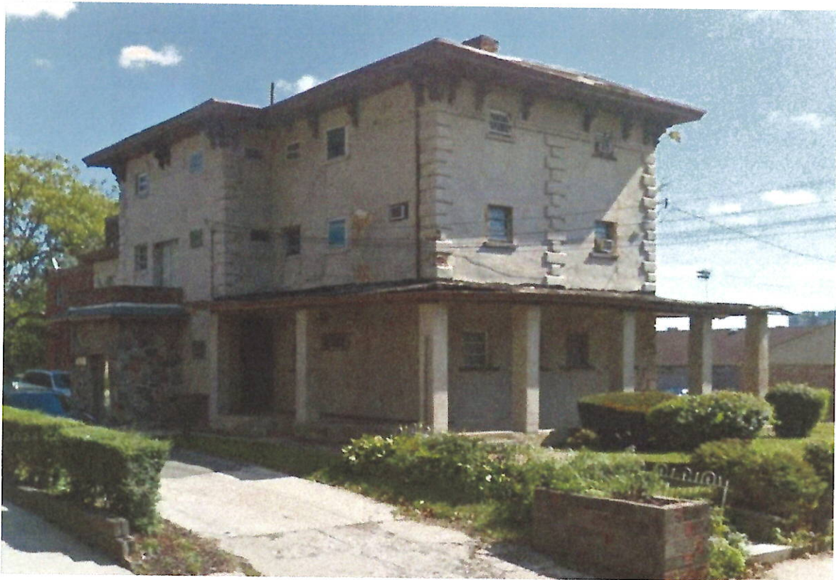
Photo # 2: showing vegetation at the roof line and spawling of the brick in the left side wall.
