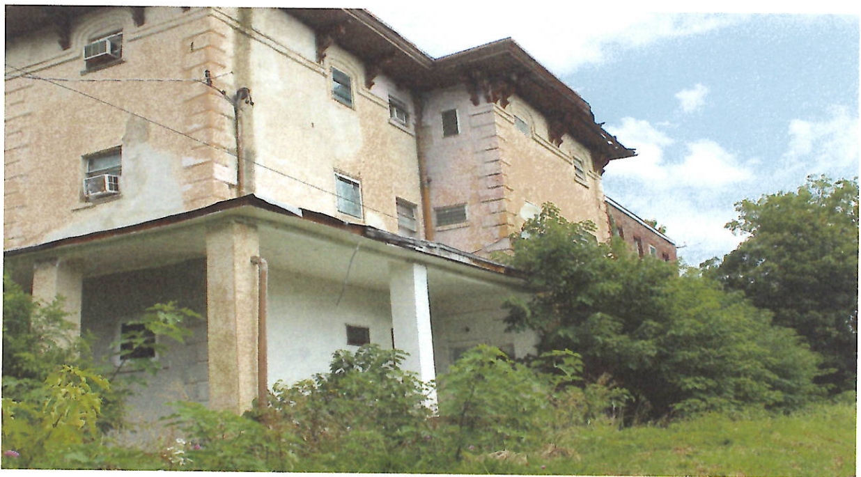
Photo # 6: showing the structural deterioration of the main roof for the building.
