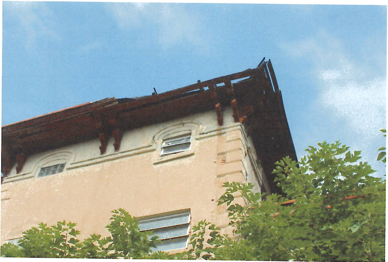
Photo # 7: showing structural deterioration of the building main roof front view.
