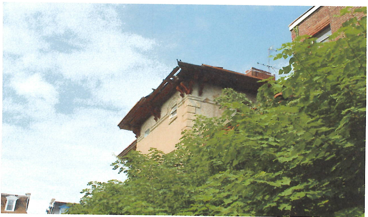
Photo # 8: showing structural deterioration of the building main roof south view.
