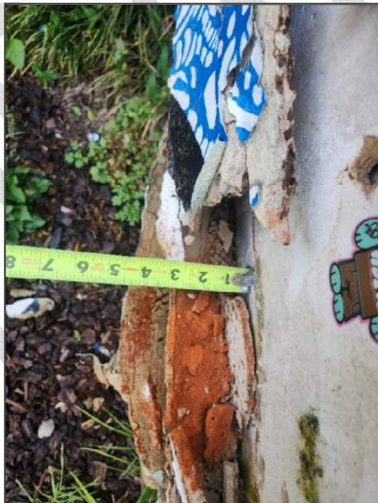
Photo No. 15: Cracked, spalled, delaminated stucco and paint; corroded metal lath at grade
