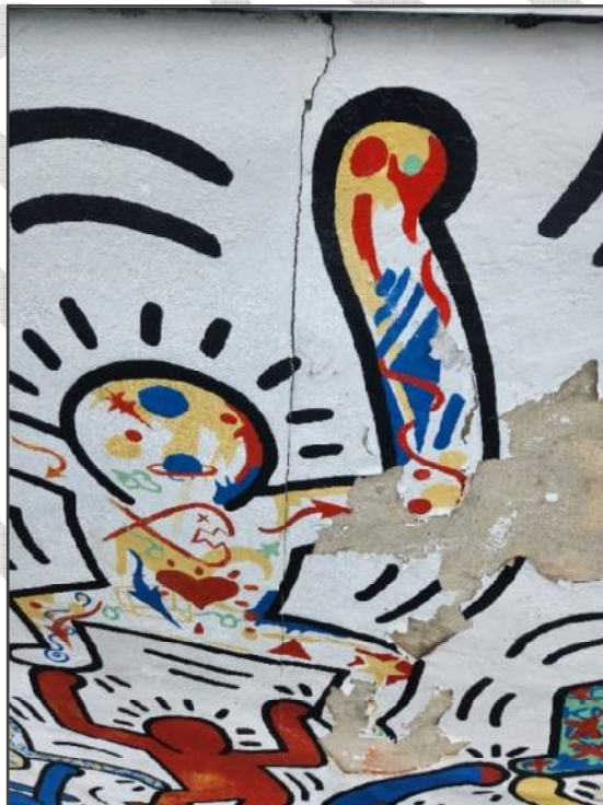
Photo No. 11: Open vertical crack through stucco at top of wall; delaminated paint
