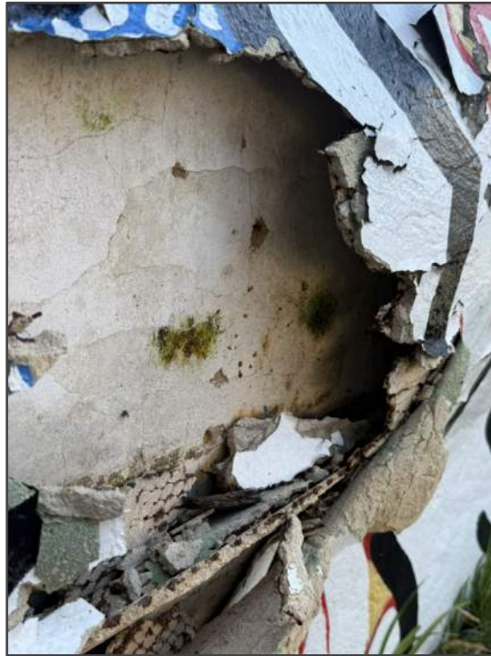
Photo No. 14: Cracked, spalled, delaminated stucco and paint; corroded metal lath at grade
