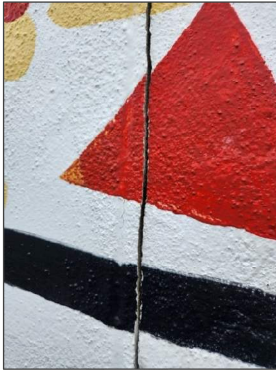
Photo No. 12: Open vertical crack through stucco
