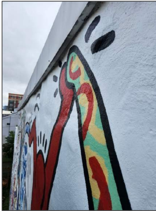
Photo No. 6: Bulging at top of wall
