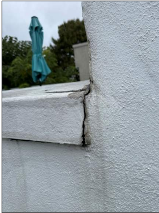
Photo No. 4: Bottom of vertical transition – joint open at end of roof deck coping
