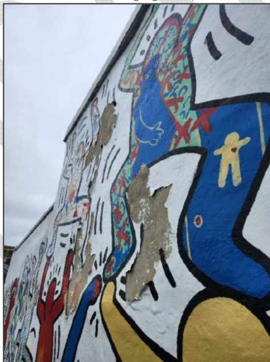
Photo No. 7: Delaminated, missing paint
