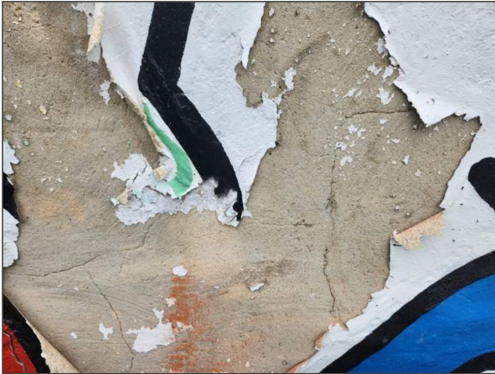
Photo No. 8: Delaminated, missing paint, cracks in stucco beyond
