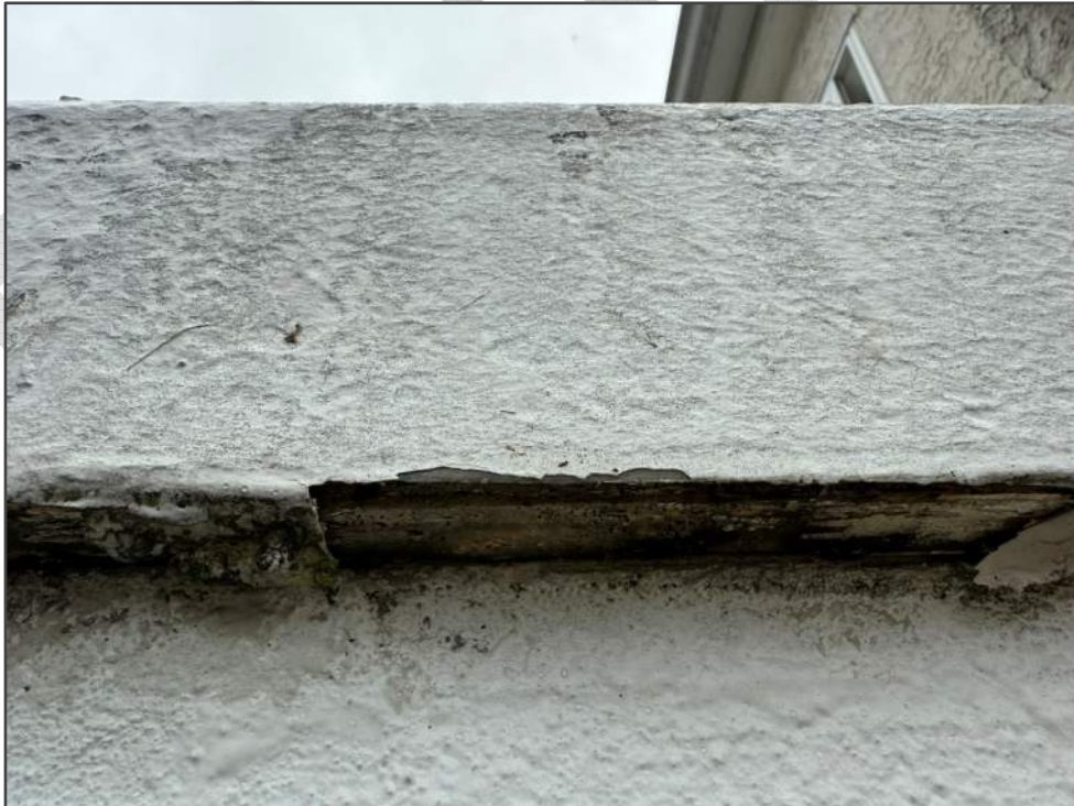
Photo No. 5: Coating flaking off underside of wood blocking at roof deck coping
