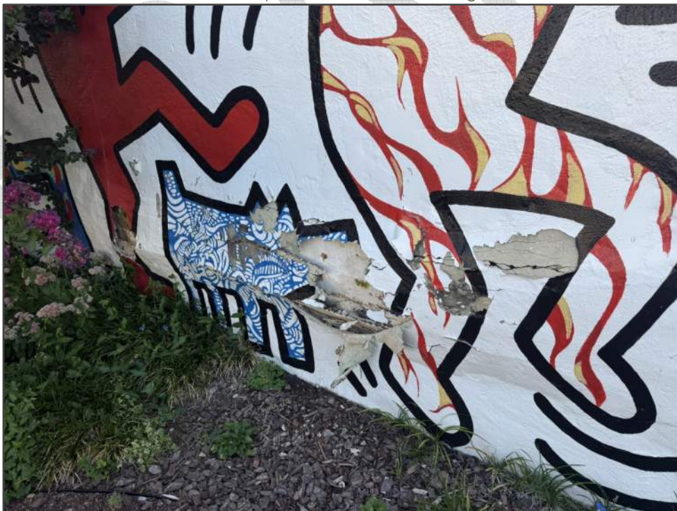
Photo No. 13: Cracked, spalled, delaminated stucco and paint; corroded metal lath at grade
