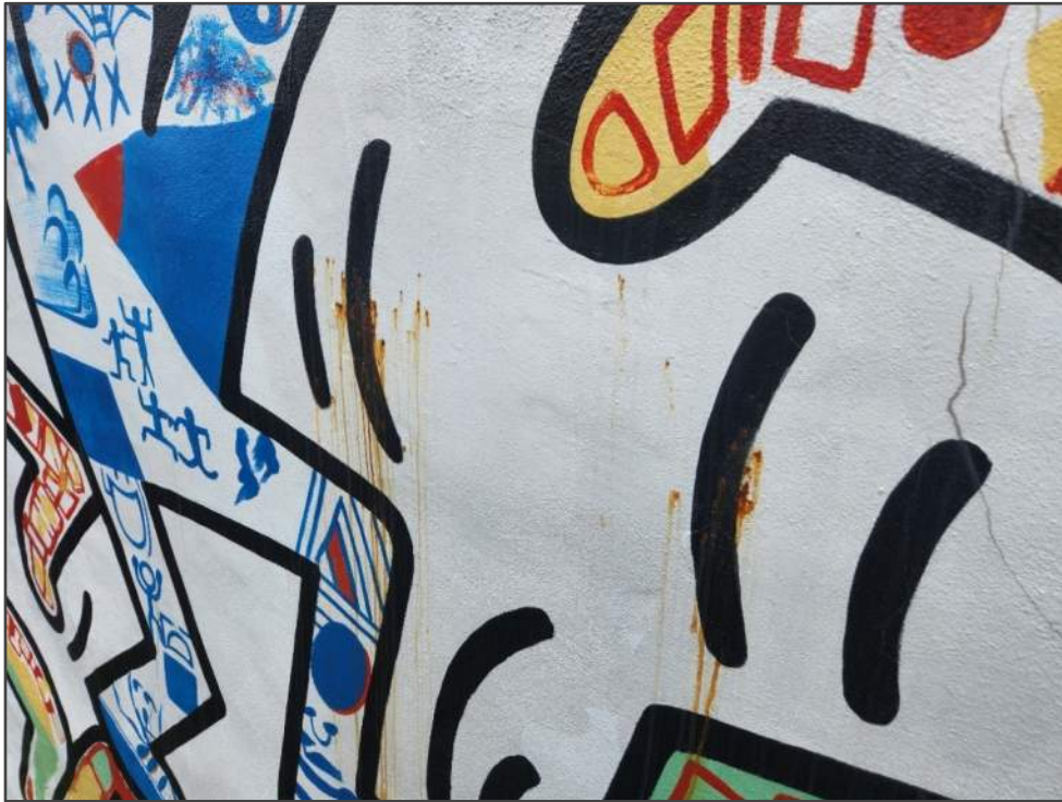
Photo No. 10: Rust staining, cracking
