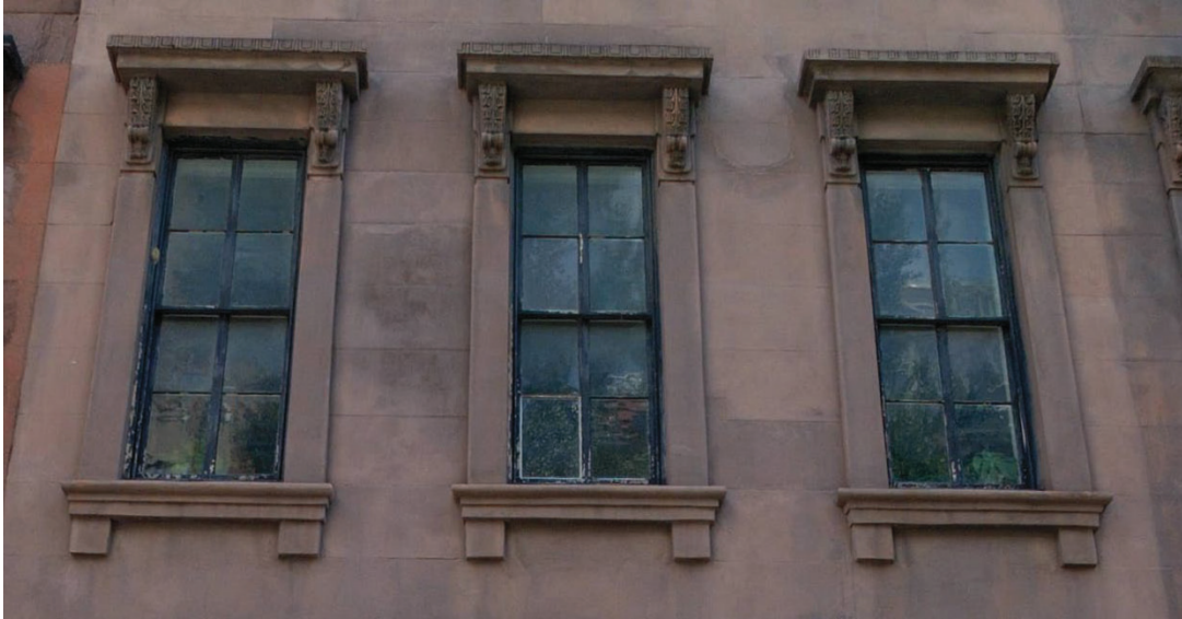
Figure 7: Surviving second-floor detail at 1522 Pine Street.
