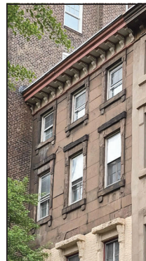
Photo C May, 2026 Detail of Upper Facade Conditions
