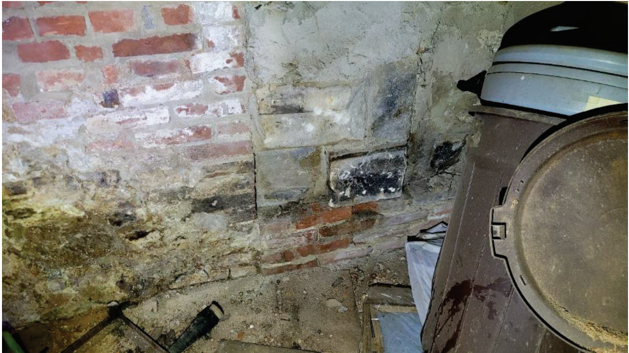
Photo No. 21. View of the deteriorated sections of the front foundation wall
