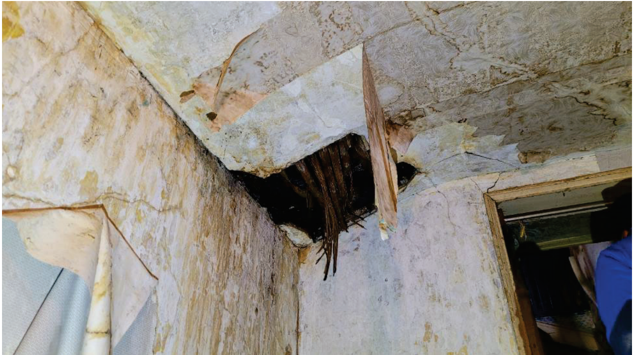
Photo No. 27. View of the rotted roof along the middle of the building, above the interior staircase
