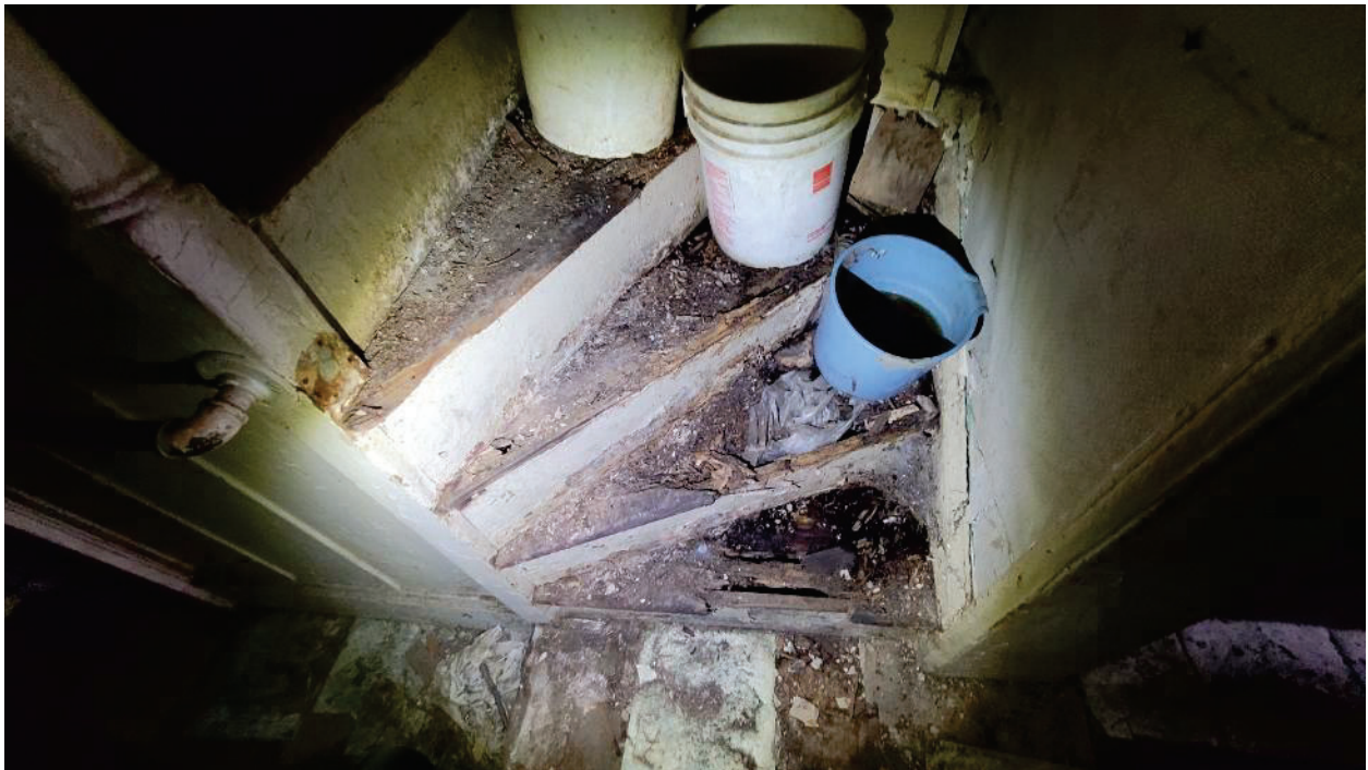
Photo No. 28. View of the significantly rotted staircase due to prolonged water exposure
