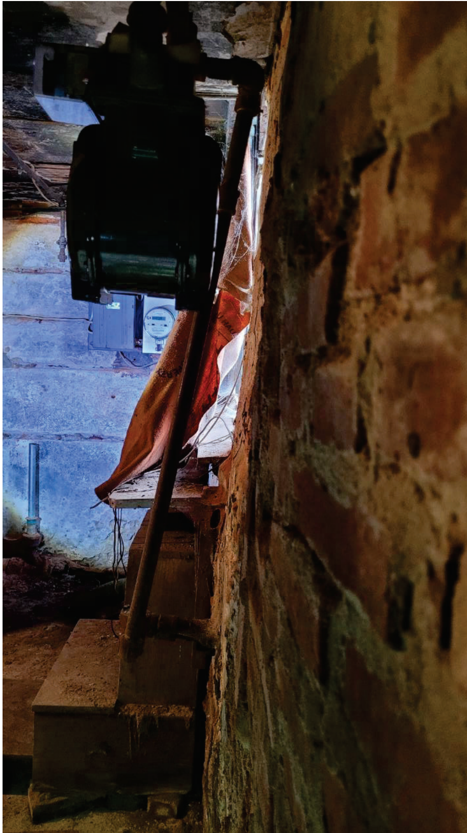
Photo No. 20. View of the significant leaning of the front foundation wall
