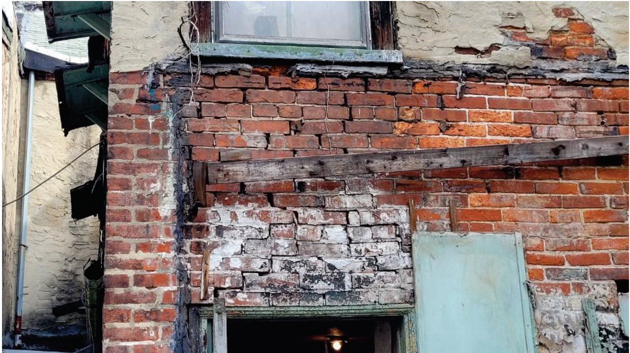
Photo No. 25. View of the decrepit exterior brick masonry of the rear wall
