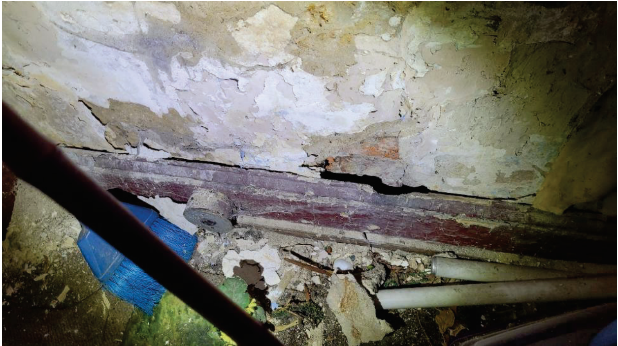
Photo No. 14. View of the deteriorated interior plaster of the 1 st floor front wall
