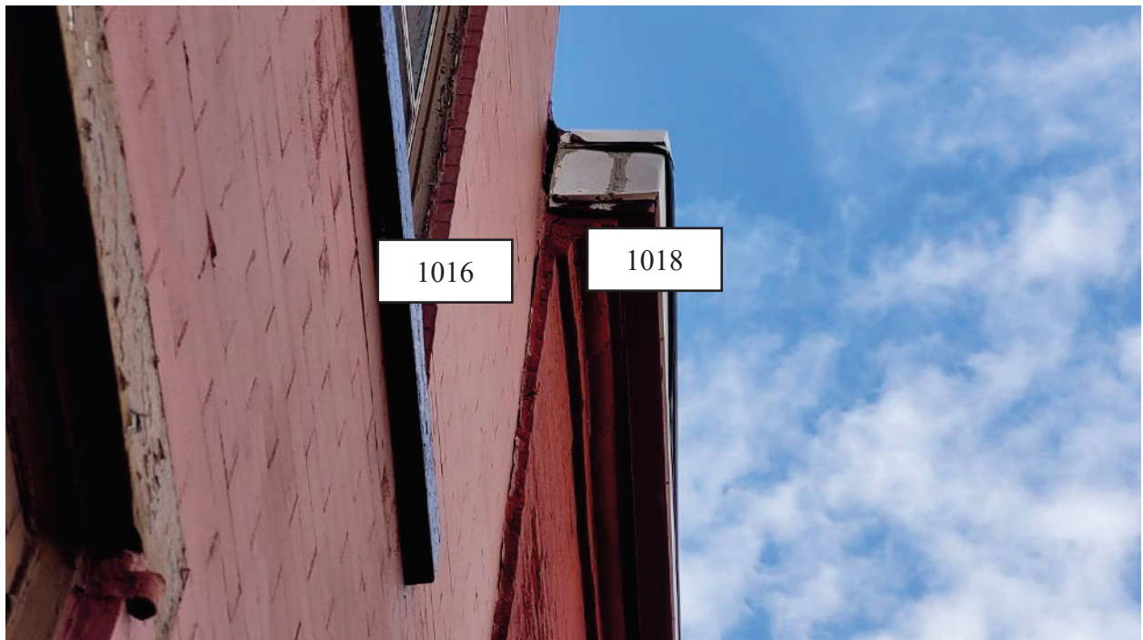
Photo No. 4. View of the upper portion of the front walls showing 1018 leaning outward relative to 1016
