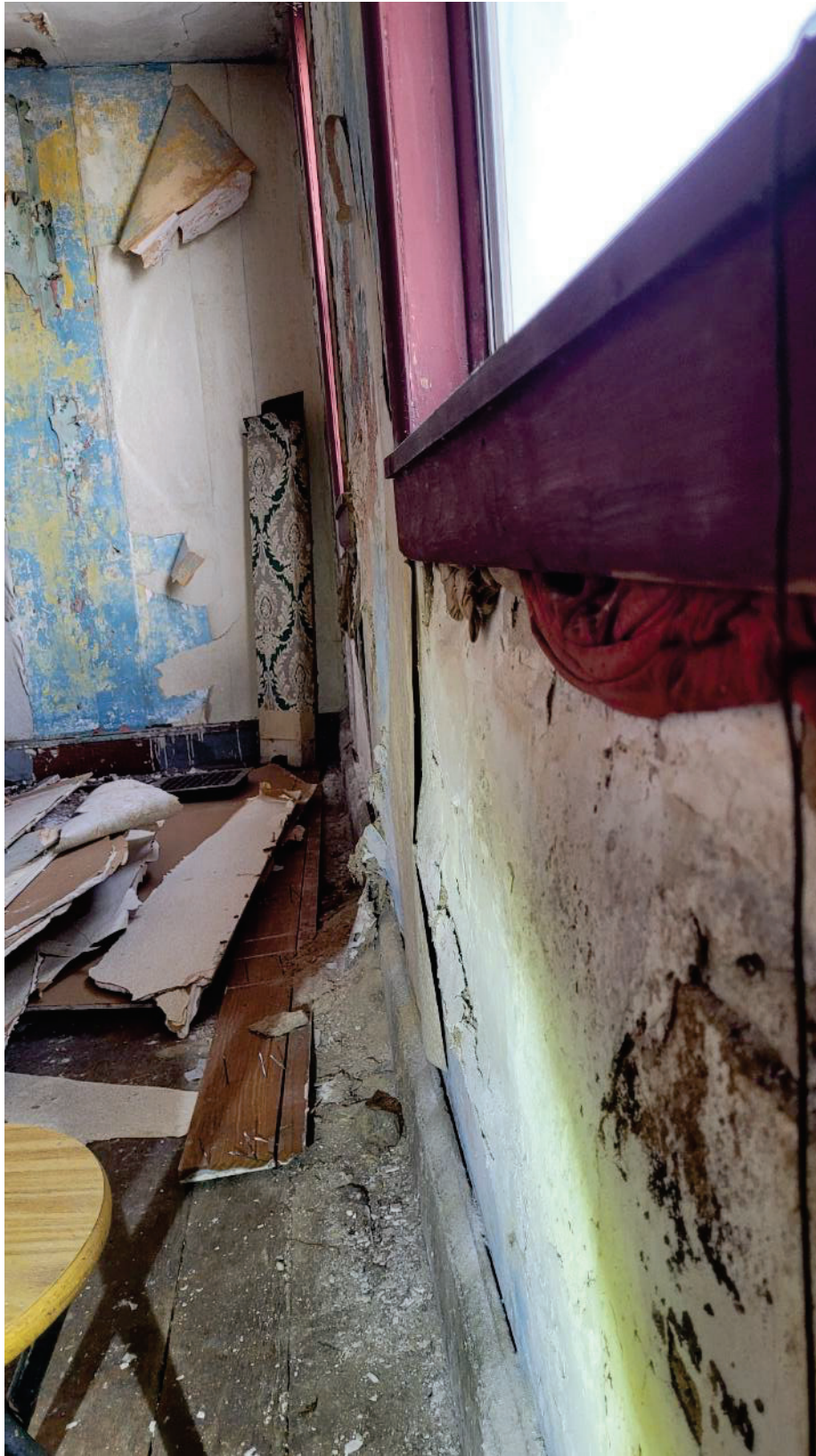
Photo No. 5. View of the significant leaning of the interior 2 nd floor front wall
