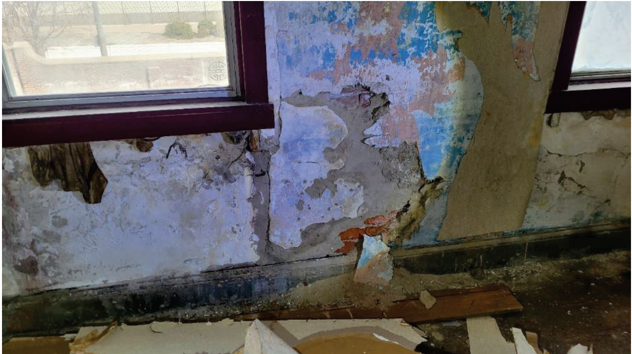
Photo No. 18. View of the deteriorated interior plaster of the 2 nd floor front wall
