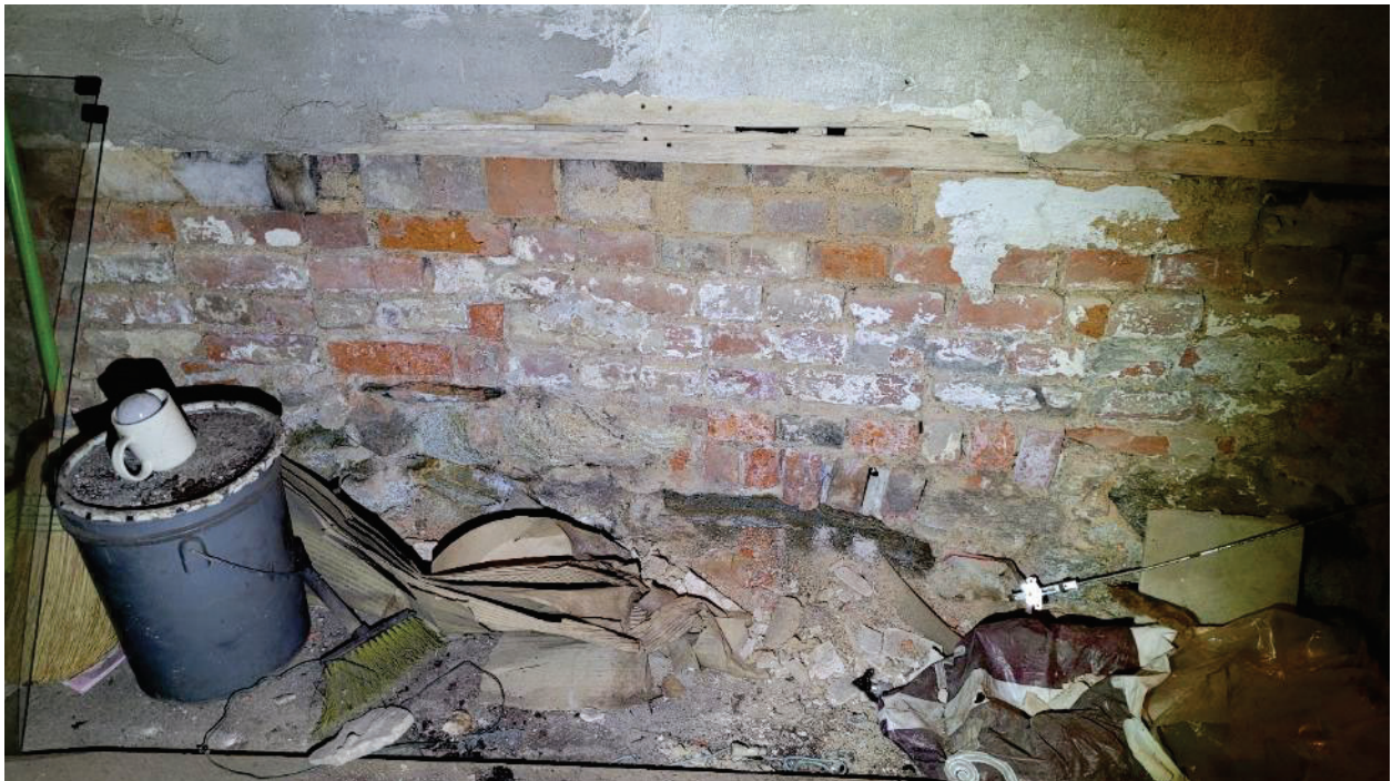
Photo No. 24. View of the decrepit foundation wall of the side load-bearing walls
