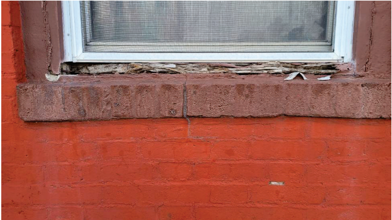
Photo No. 8. View of the cracked and sagging 1 st floor windowsill
