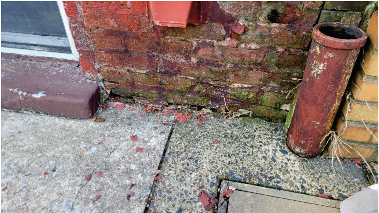
Photo No. 11. View of the decrepit and deteriorated brick masonry throughout the front façade
