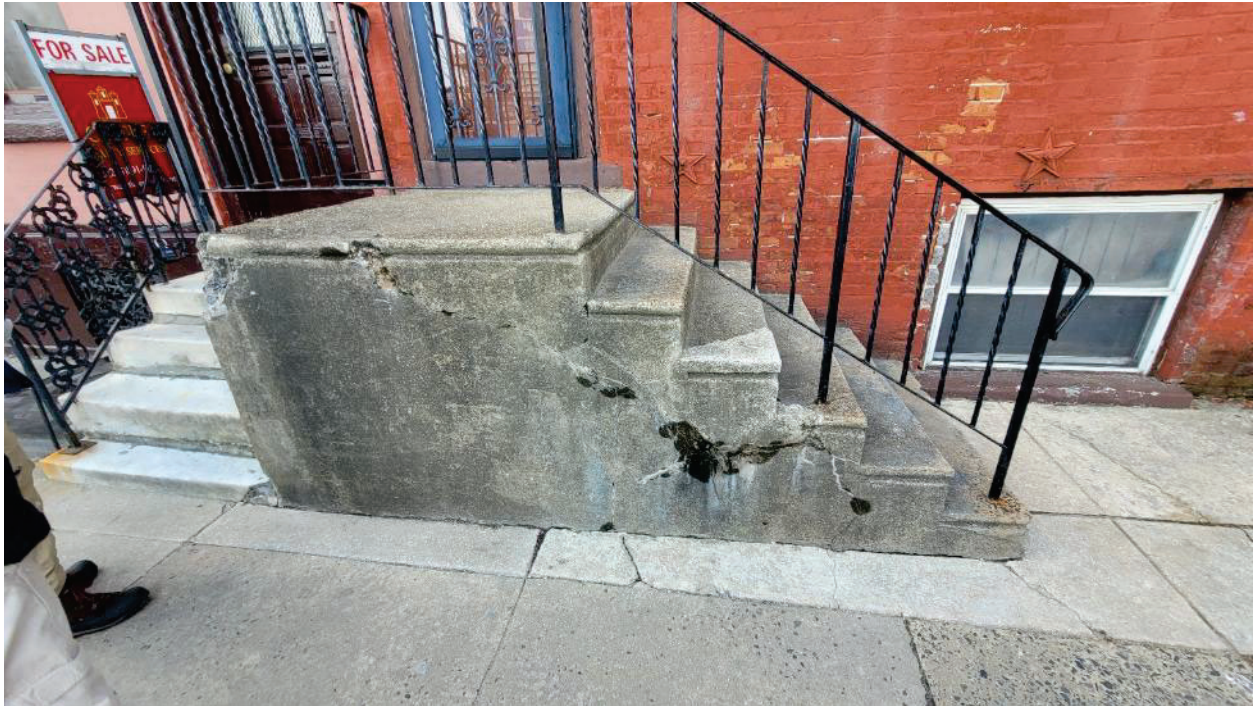
Photo No. 23. View of the concrete steps at the front door with section loss and cracking throughout
