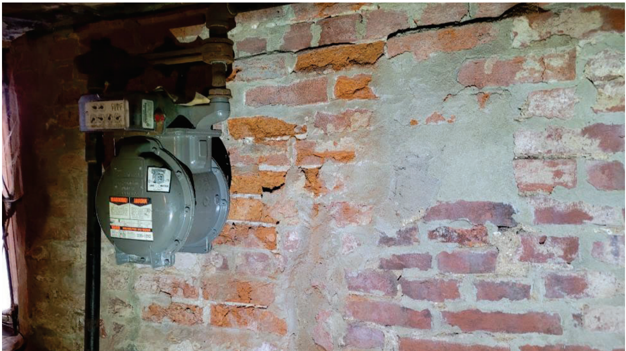
Photo No. 22. View of the deteriorated sections of the front foundation wall
