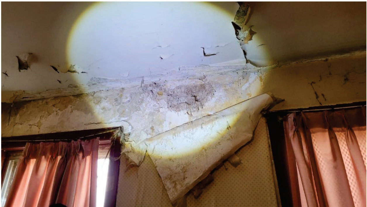
Photo No. 13. View of the deteriorated interior plaster of the 1 st floor front wall
