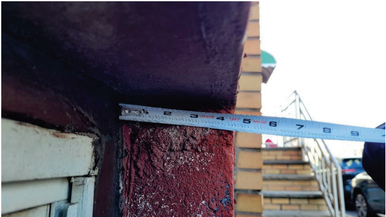
Photo No. 7. View of the measured distance from the basement window frame to the front wall at the top of the window (approximately 4-1/4 inches)
