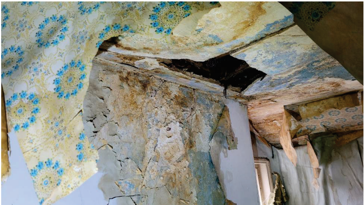
Photo No. 26. View of the rotted roof along the rear of the building
