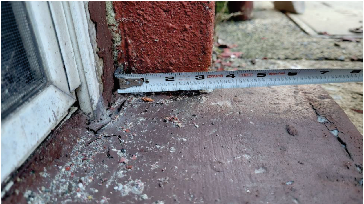
Photo No. 6. View of the measured distance from the basement window frame to the front wall at the bottom of the window (approximately 3-1/8 inches)
