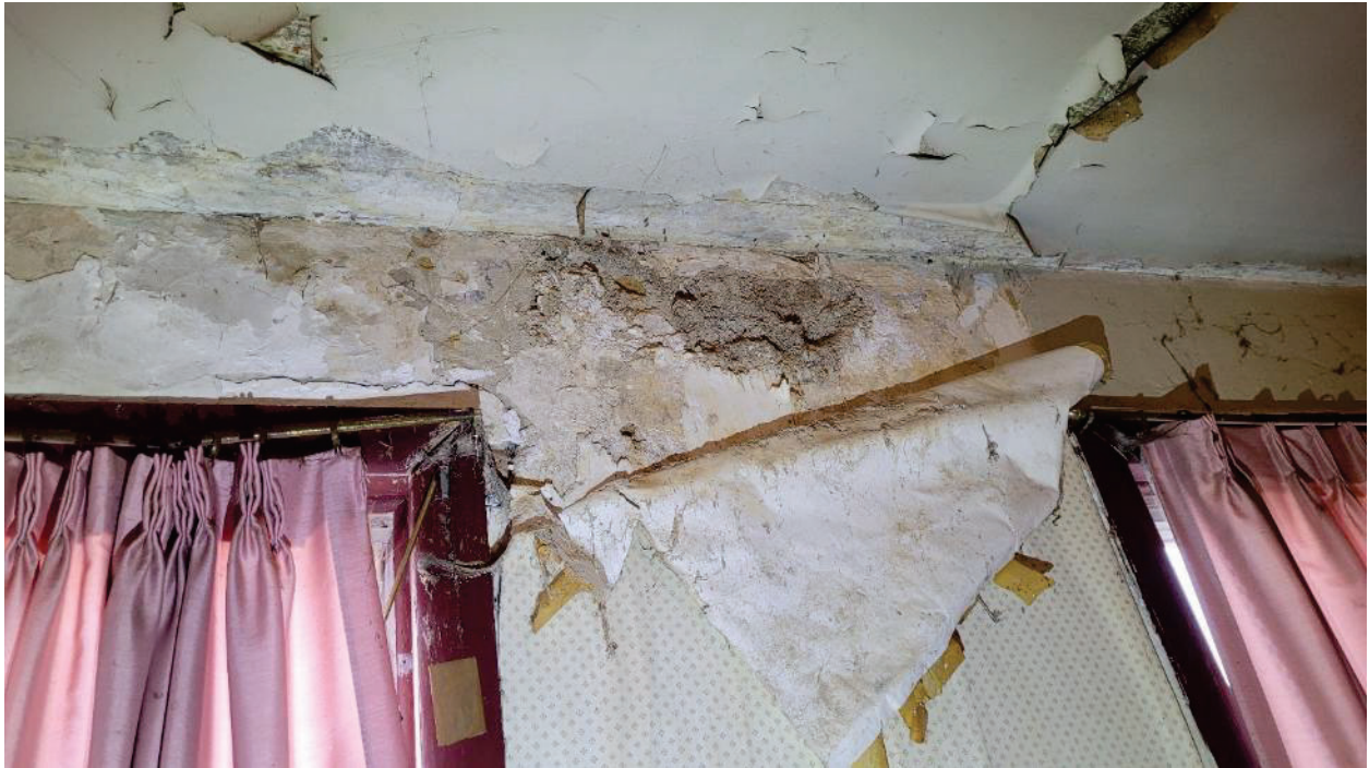
Photo No. 16. View of the deteriorated interior plaster of the 1 st floor front wall
