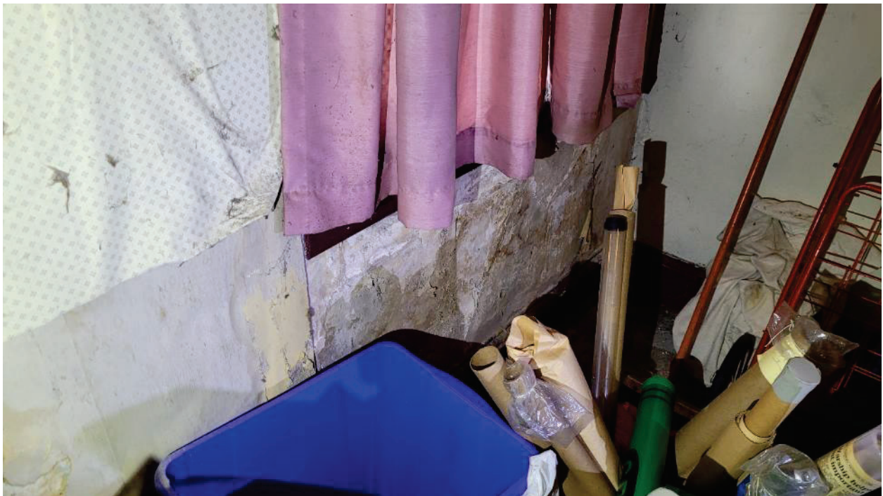
Photo No. 15. View of the deteriorated interior plaster of the 1 st floor front wall
