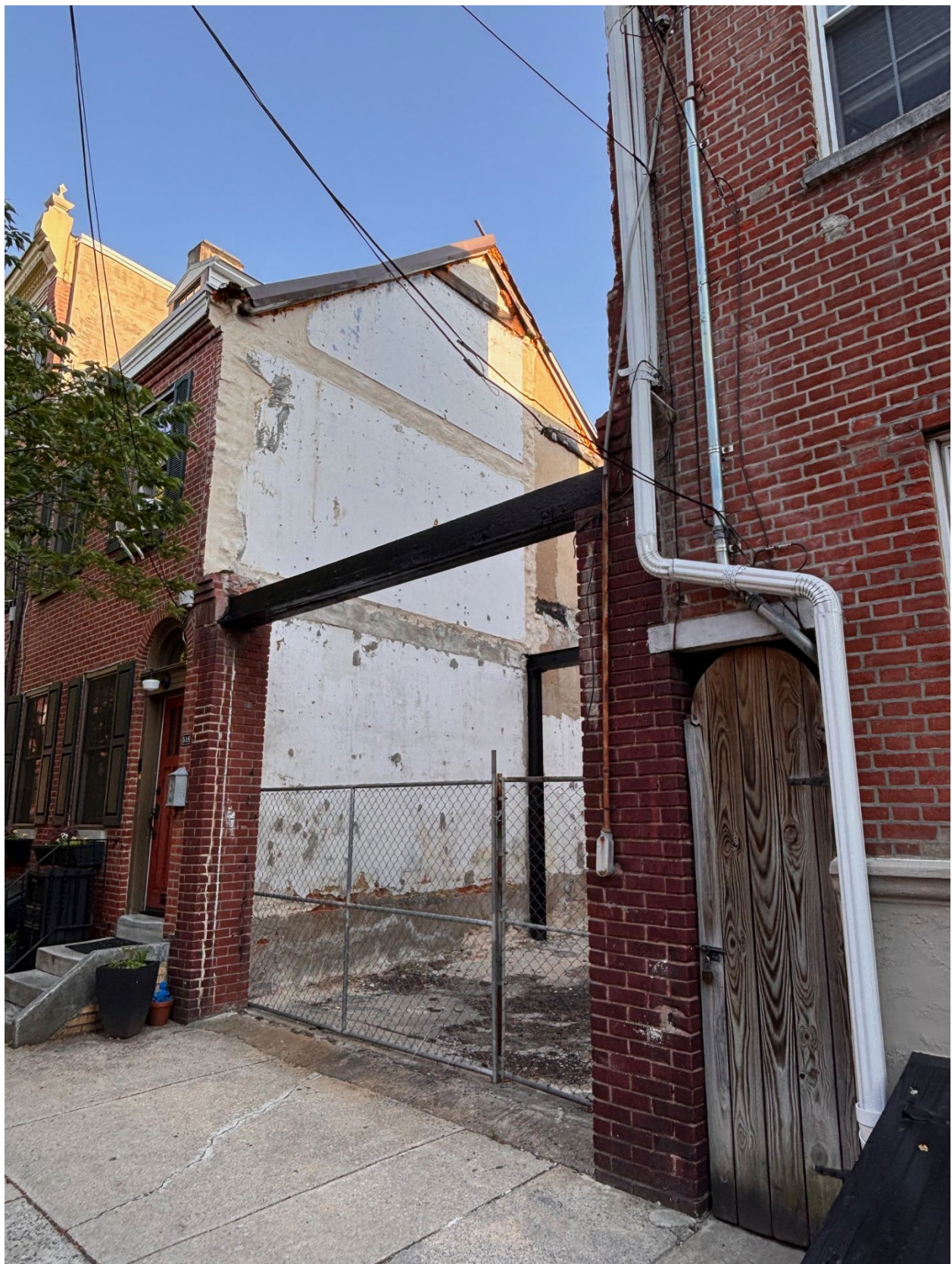
Figure 7. 520 Queen Street, April 23, 2026.
