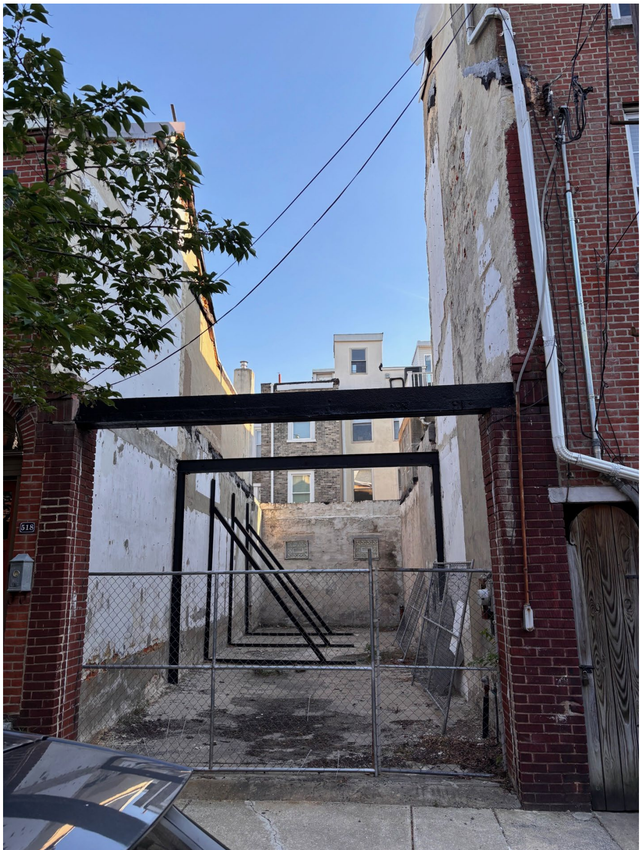
Figure 6. 520 Queen Street, April 23, 2026.
