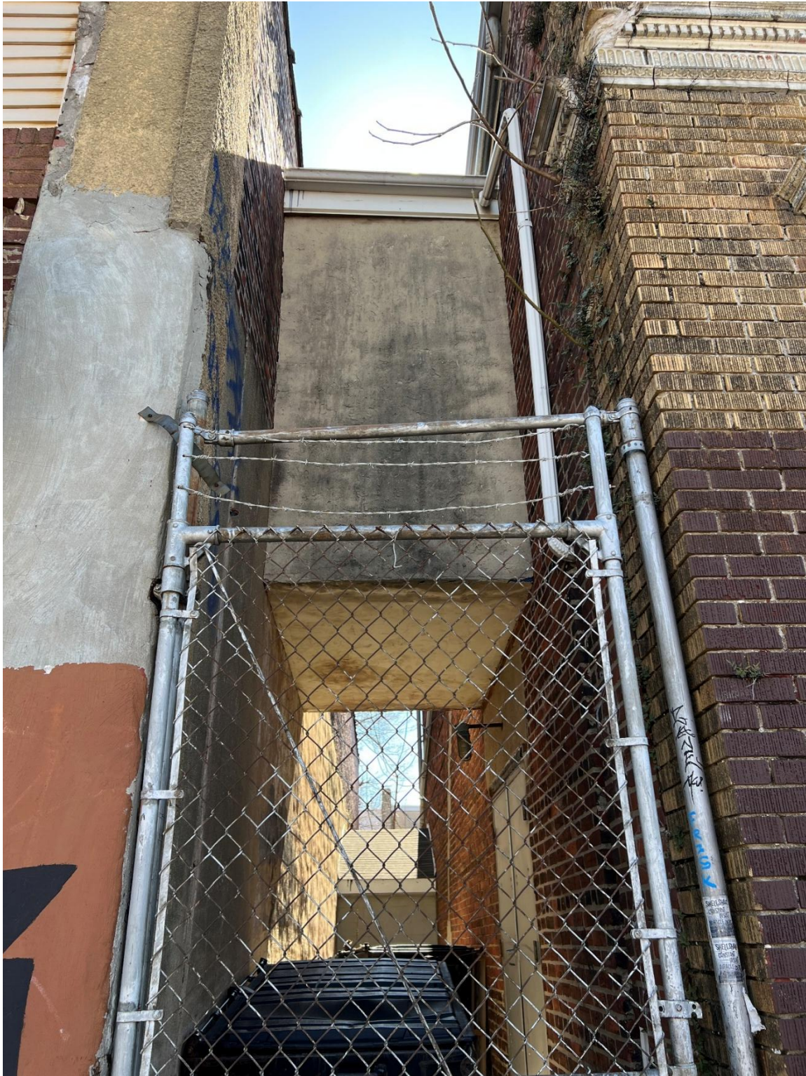
Figure 23: View of the east elevation of the Ambassador Theatre and interconnections to the adjacent building.
