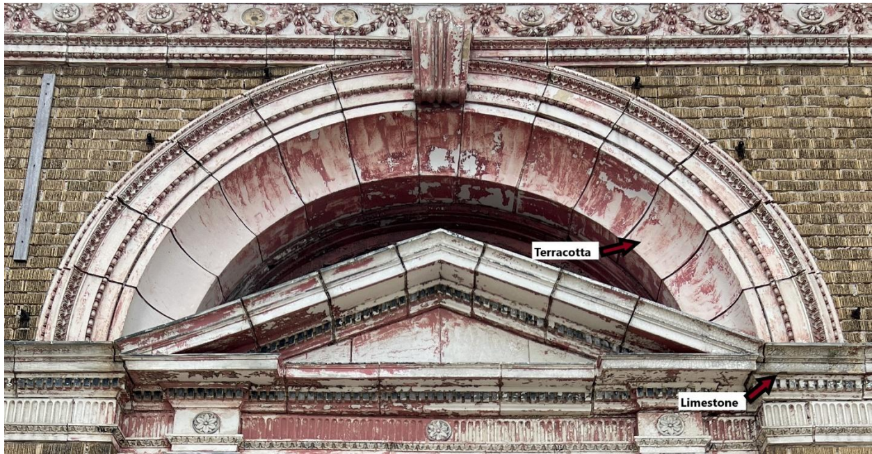
Figure 10: Detail view of the west volume's arched window, calling out the subtle difference in appearance between the terracotta and limestone ornamentation, divided by the stringcourse.
