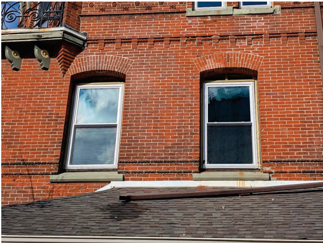
Figure 3. Close up of front façade with replacement windows and missing brickmold. May 2026.
