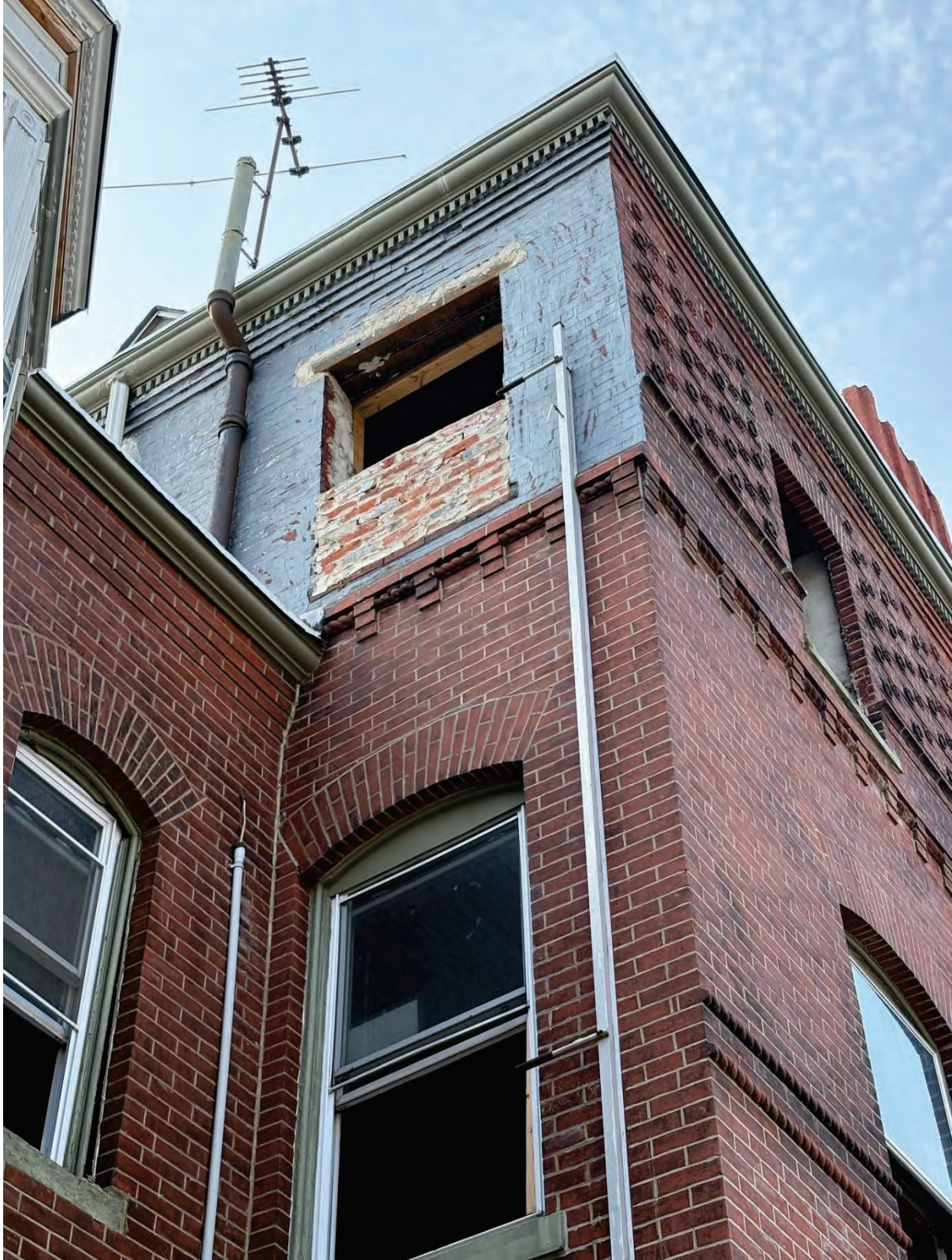
Figure 4. Prior to window replacement. Image shows build down of third floor window and lintel replacement. At this time in July 2025, original brickmold was still in place in most window openings.
