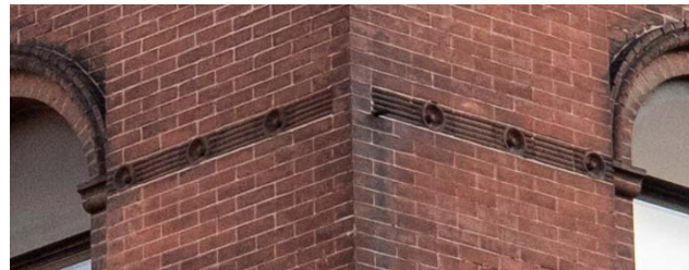
Figures 28 and 29. Terra cotta belt course, ornamental bands, and running bond brickwork
