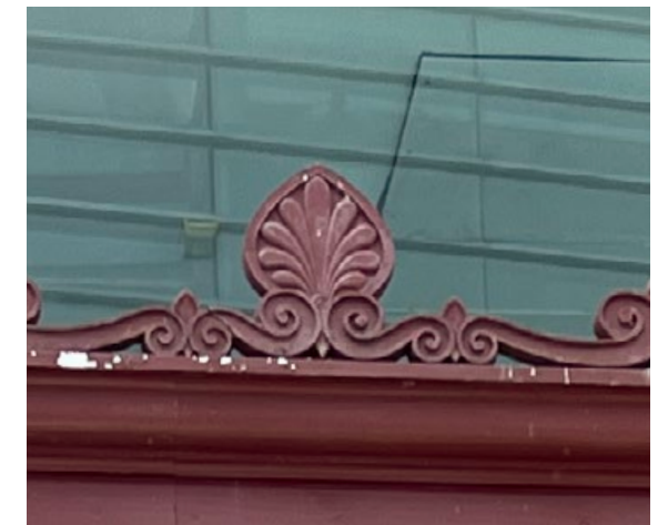
Closeup of Facade paint wear
