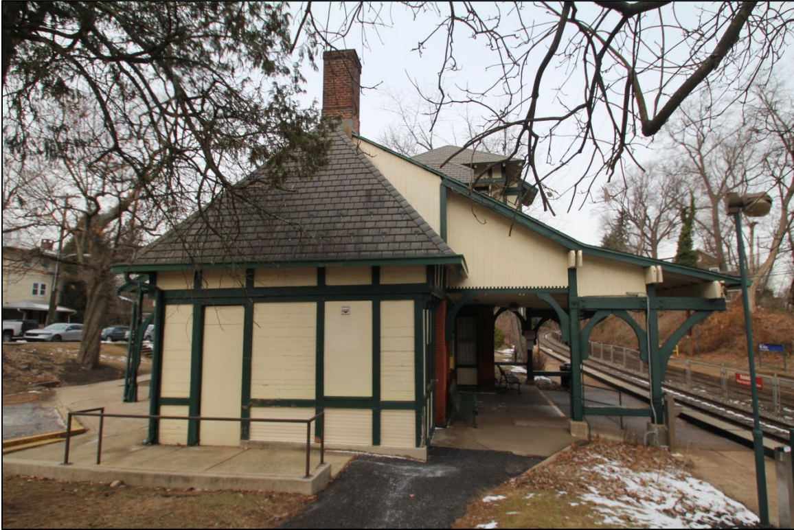
Photo 5: 119 East Gowen Ave, southeast elevation, looking northwest. The change in slope of the roof leading from the station to the platform is clearly visible. (Robert Powers, 2025)
