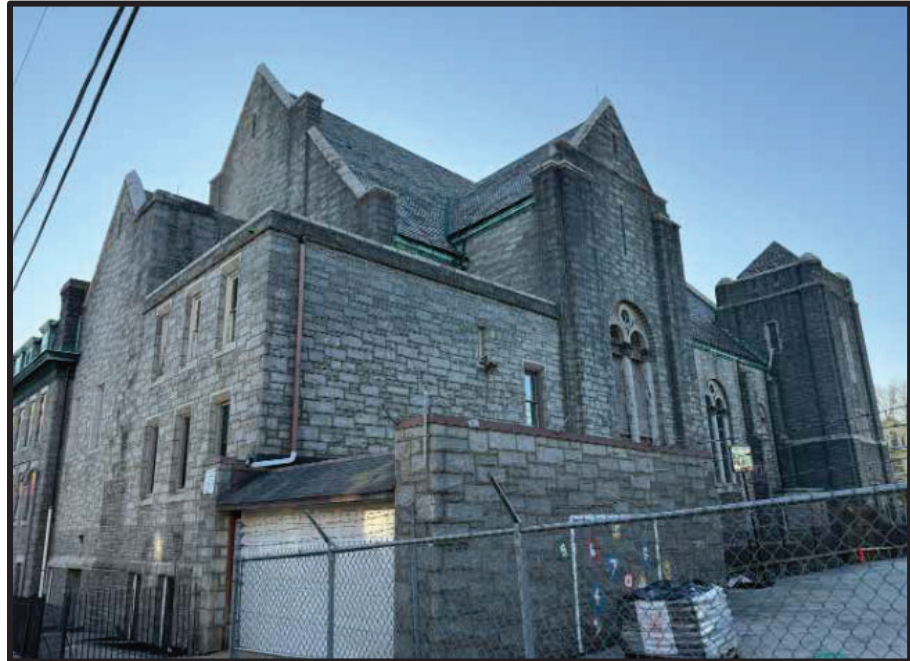
Figure 6. Top: The side (northeast) elevation. Figure 7. Bottom: The side (northeast) and rear (southeast) elevations. Source: Oscar Beisert, 2026.
