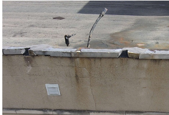
Replace damaged coping stone
