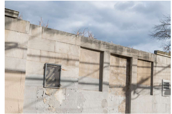
Replace missing cornice
