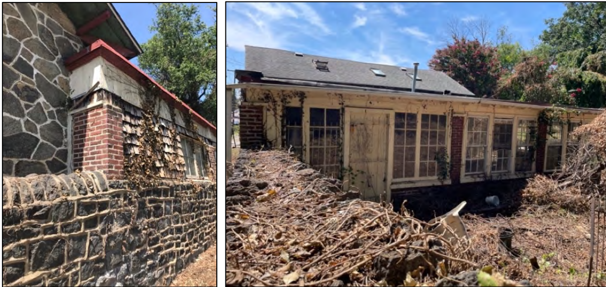
Fig. 22, left. The north walls of the stone building and the solarium intersect with each other, and the solarium wall rises from the perimeter schist wall. Fig. 23, right. The north wall of the solarium showing the extensive fenestration along this elevation with low sills in the brick wall and a couple of brick pilasters breaking up the window openings. An access door is located closer to the east side of this elevation. The roof field of the stone building beyond can be seen with skylights. Far left foreground is the top of the perimeter schist wall. Photos: August 9, 2025.
