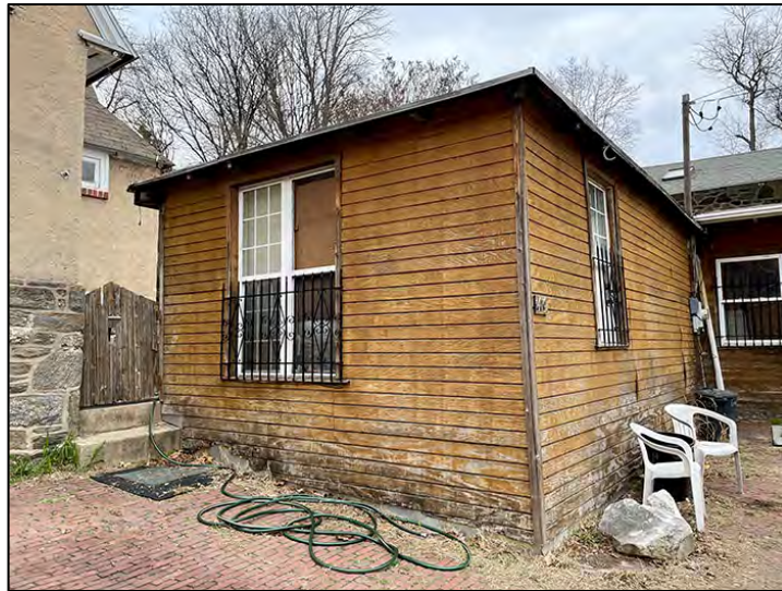
Fig. 17. The south and east elevations of the workshop portion of the garage. This leg of the L-shaped construction extends toward the cottage (left side) into the brick motor court. The wood gate on the left between the garage and the cottage leads from the motor court to the garden. Date: March 28, 2025.
