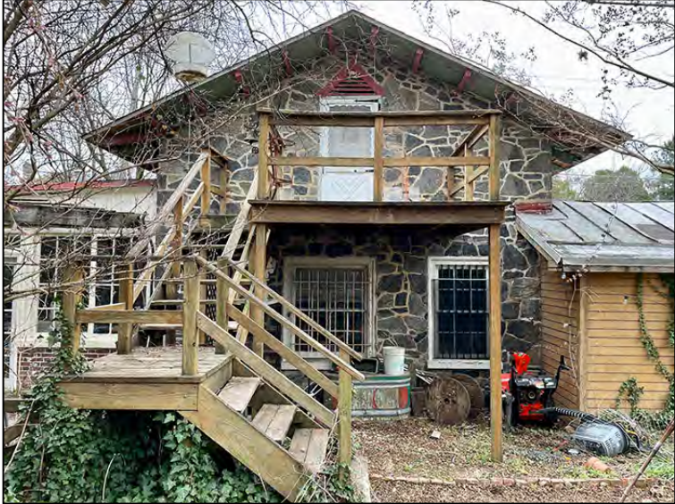
Fig. 21. The west elevation of the stone building facing the garden and showing the connections to the garage to the south (right) and to the solarium to the north (left). There are two window openings at the lower level which do not appear to have been altered from door structures; each contains wood frames and divided lite windows. Date: March 28, 2025.
