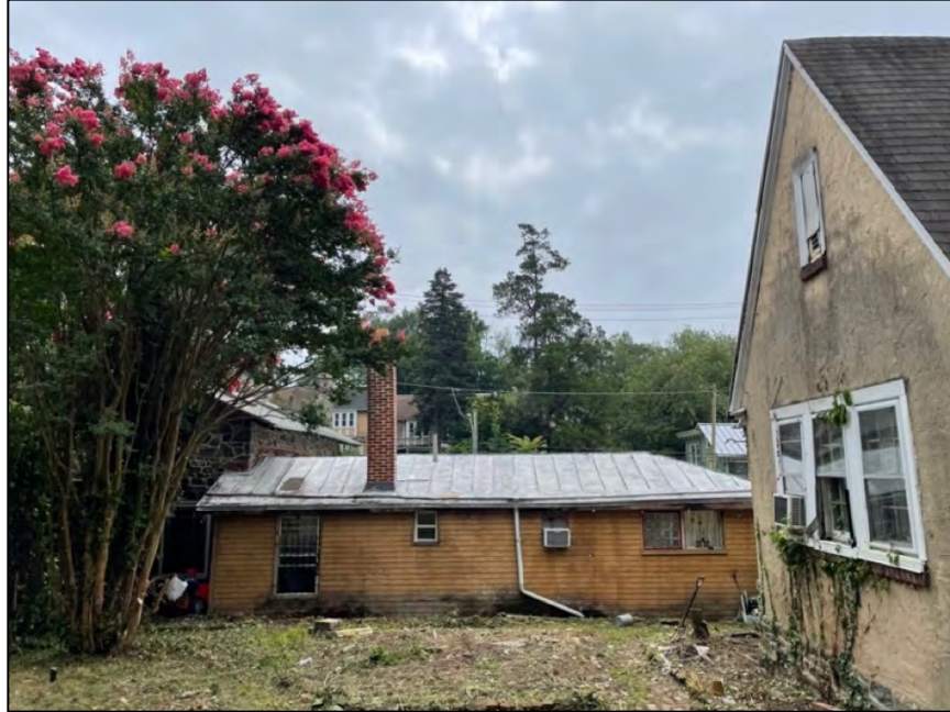
Fig. 14. West elevation of the garage's workshop, taken from the garden. Date: July 27, 2025.
