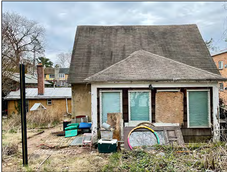
Fig. 9. West elevation of the 1923 Cottage. Note the brick footpath that extends from the motor court access gate along the north side of the building and around to the rear lean-to. Date: March 28, 2025.
