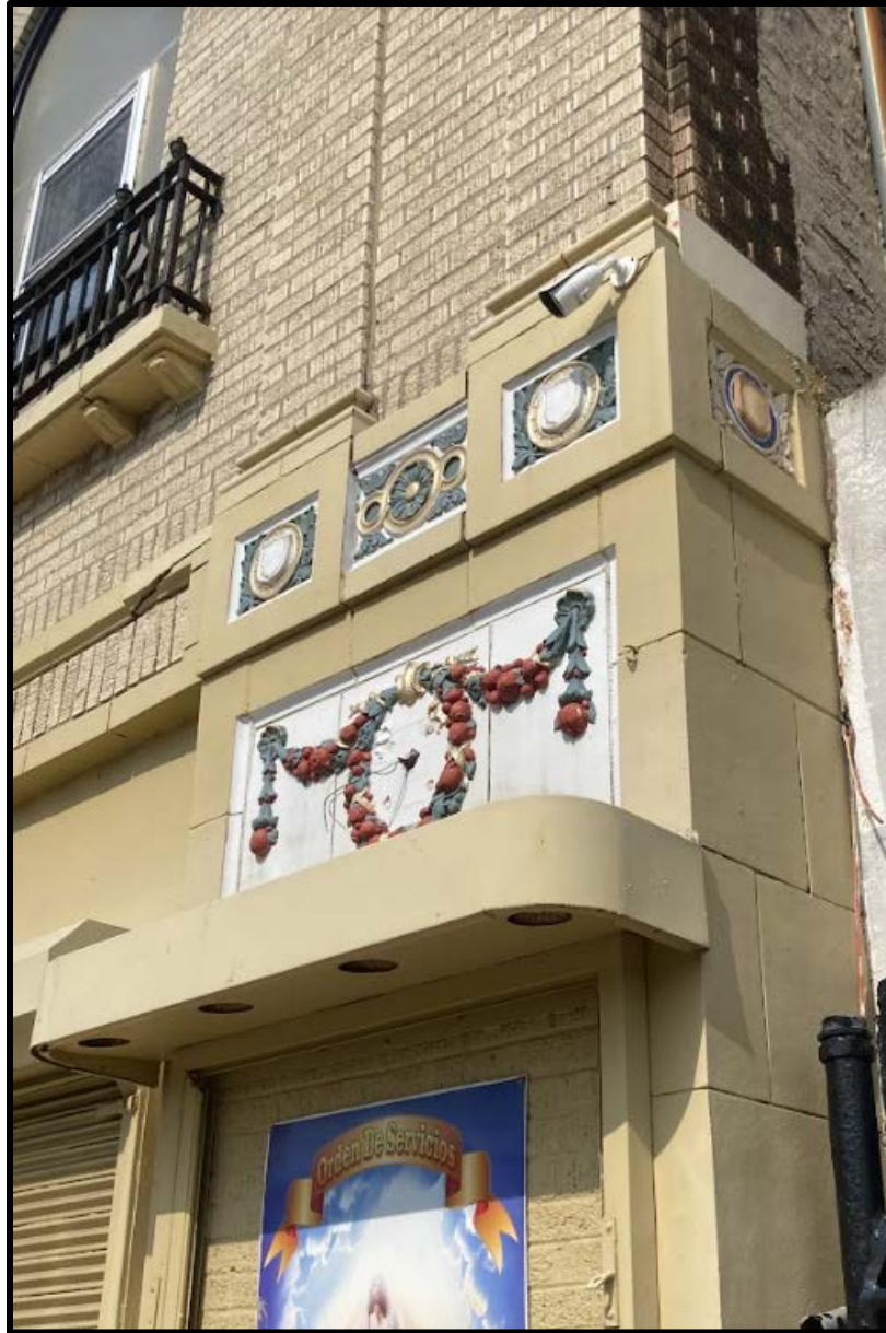
Figure 7. Architectural terra cotta at the southwest corner of the subject building. Source: Andy Molholt, 2024.
