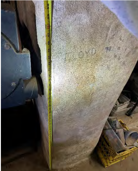
Figure 2: Highwater mark within the building for Hurricane Floyd (1999).
