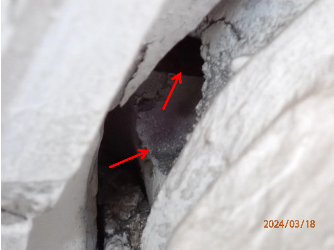
Photograph 9 – Cored hole in terra cotta flower unit and steel bar.
