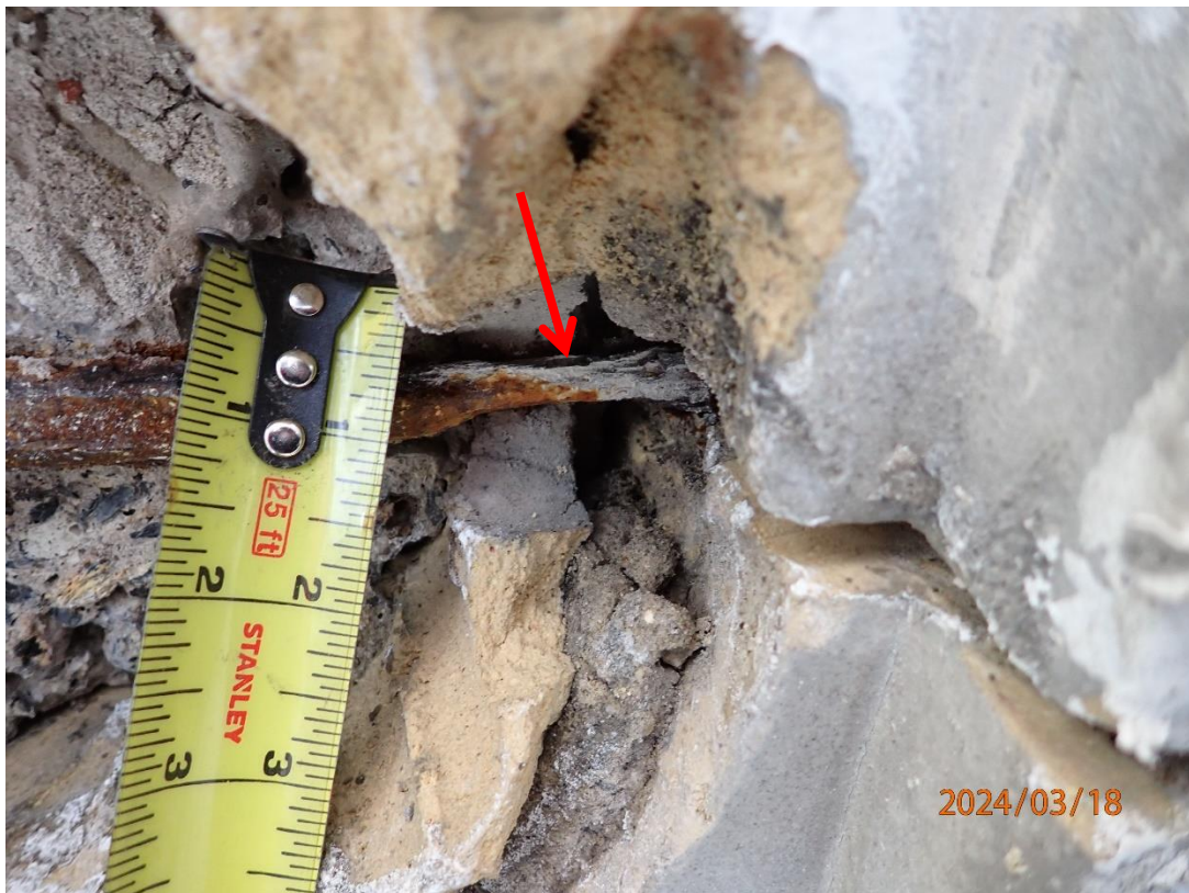
Photograph 10 – Corroded steel bar with 50% section loss.
