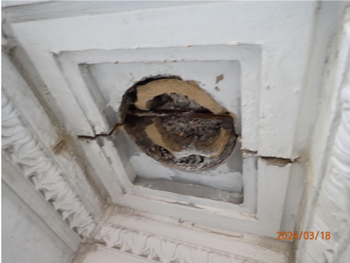
Photograph 7 – Overview of removed/fallen terra cotta flower unit.
