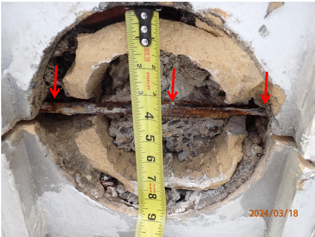
Photograph 8 – Overview of terra cotta flower unit support, steel bar shown with red arrow.
