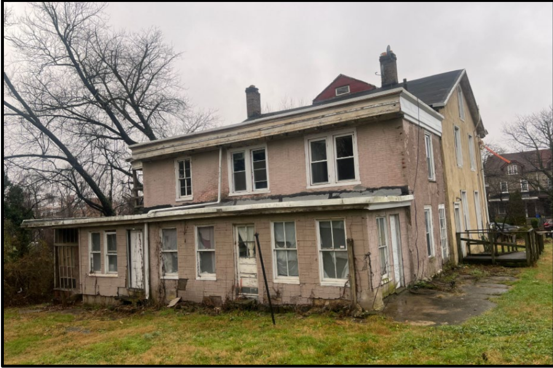
Figure 11. The Smith-Steel-Humphreys House, 424 E. Woodlawn Street, Rear (Southeast) and Side (Northeast) Elevations of the Rear Brick and Rear Frame Additions. Source: Oscar Beisert, 2023.
