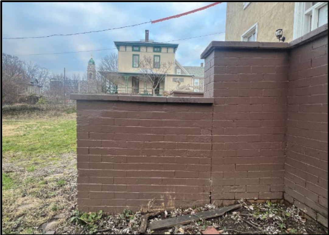
Figure 7. Top: A photograph by Phebe Westcott Humphreys of her plants on the brick supports of the front steps of the subject house in 1905. Source: Phebe Westcott Humphreys Collection, HSP. Figure 8. Bottom: The brick supports of the front steps to the subject house, as shown in the 1905 photograph.
