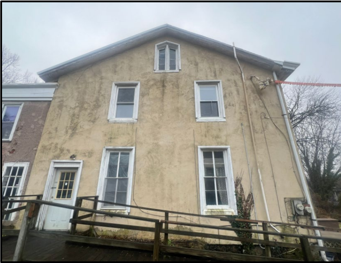
Figure 9. The Smith-Steel-Humphreys House, 424 E. Woodlawn Street, Side (Northeast) Elevation of the Main Block. Source: Oscar Beisert, 2023.
