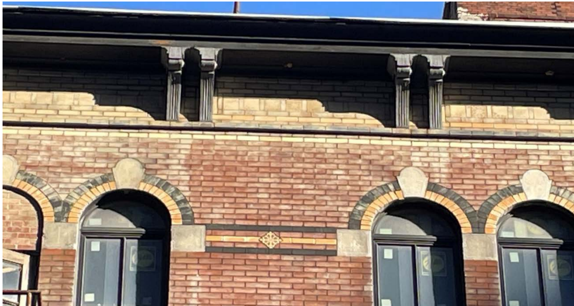
Figure 39: Detail showing the fourth-floor ornament as well as the cornice, which features a band of tiles as well as several courses of colored bricks. This elevation was previously painted, obscuring some of the flourishes.
