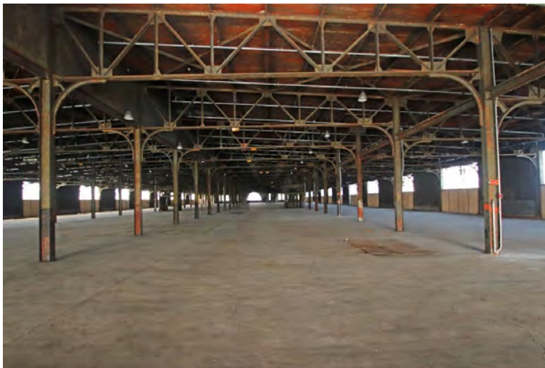
Photo 15: Second story of Pier 38, looking west. In this view, one of the original floor hatches, which consist of double steel doors that swing open, can be seen next to the columns on the right side.
