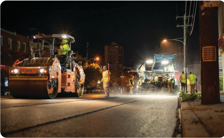
Steam rises off fresh asphalt under the glow of work lights as paving crew workers operate heavy machinery during overnight street resurfacing on Washington Avenue.
