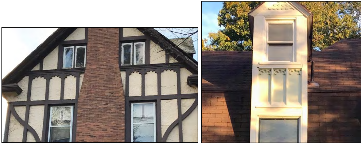
Figs.26 & 27. The spandrel panels between the 2 nd and 3 rd floors of the south elevation of Overleigh and the north elevation of the 1886 Primrose Cottage that face each other. These houses are two George T. Pearson designs on McKean Avenue in Germantown.
