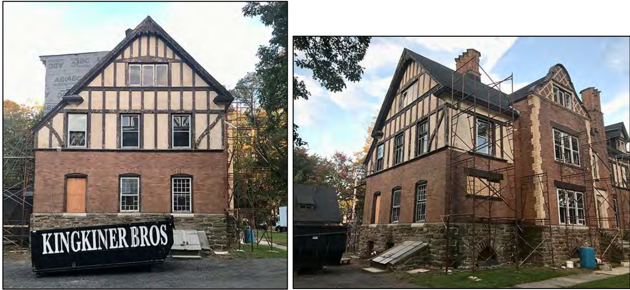
Figs. 13 & 14. Left, the north elevation showing the half timbering at the upper levels and the side of the new egress dormer at the third level apartment. Right, the northwest corner of the house showing the service side including a basement bulkhead. Both photos, October 13, 2023.
