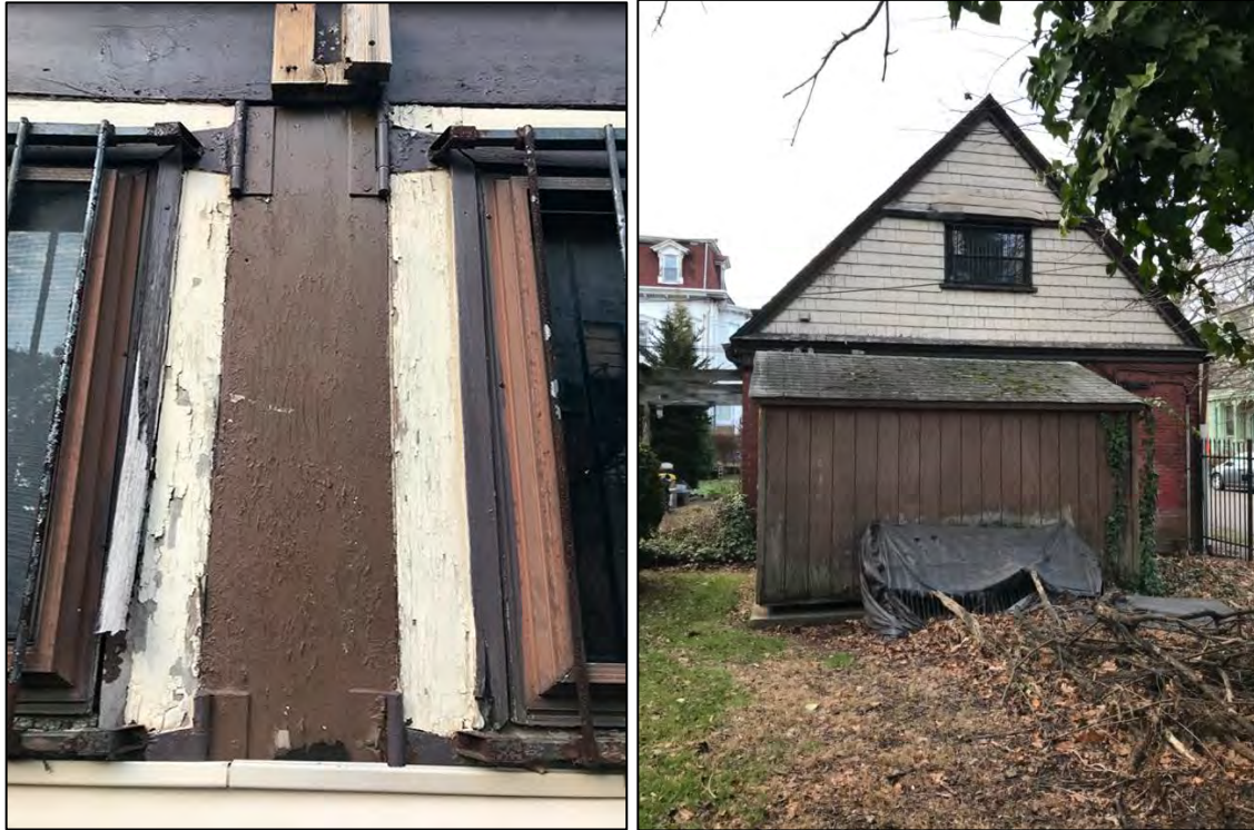
Figs. 16 & 17. Left, hinges at the three garage openings at the west elevation are intact. Right, the south elevation of the garage with a window in the second level gable and a storage shed in front. October 13, 2023.
