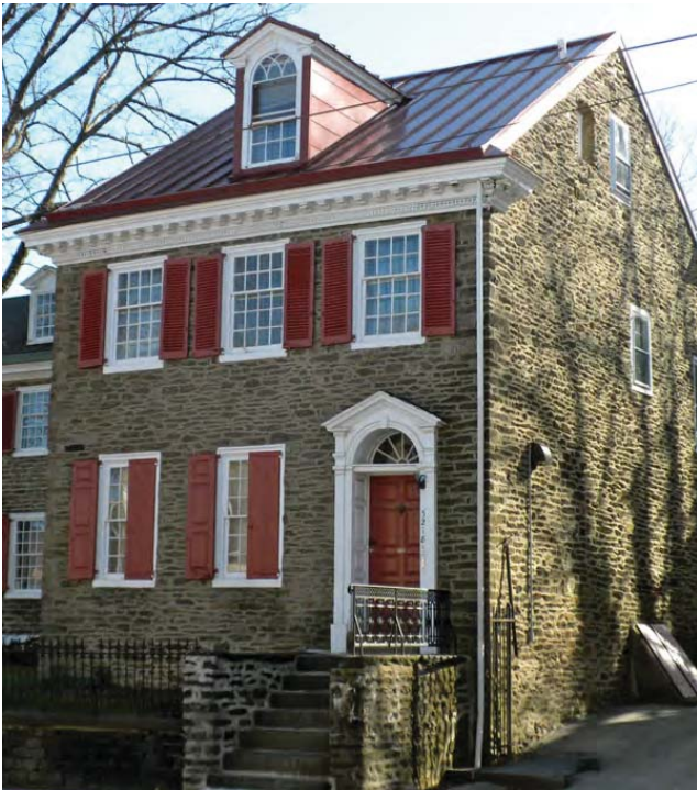
5208 Germantown Avenue Side wall: rubble with long & short corner Window frames support masonry
