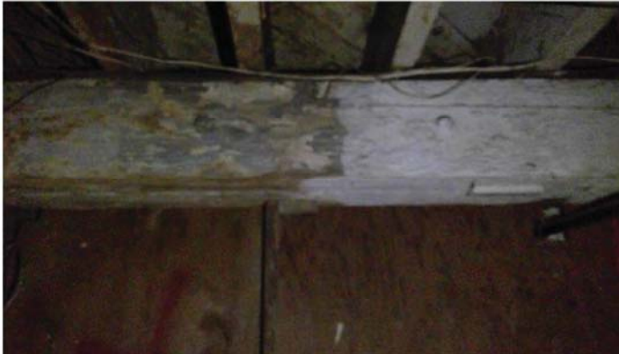
Structural deterioration in basement
