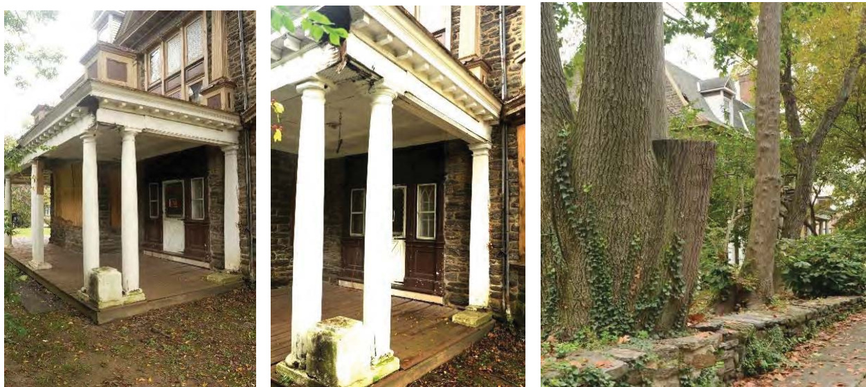
Missing porch columns; missing porch railing; failing porch deck; jury-rigged porch post supports; holes in main house roof
