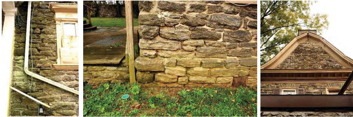
Pointing and masonry conditions, washed out pointing and soft mortar; settling split in kitchen wing roof cornice
