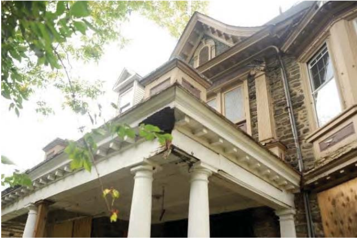
Rot in wood, missing columns, animal holes in cornices (August 2020).
