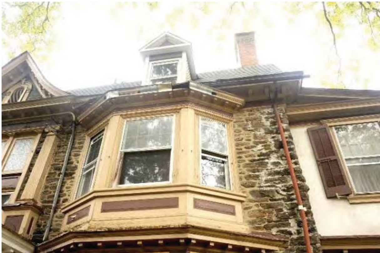
Rot in wood; missing porch railing; extensive masonry damage at second floor (August 2020)
