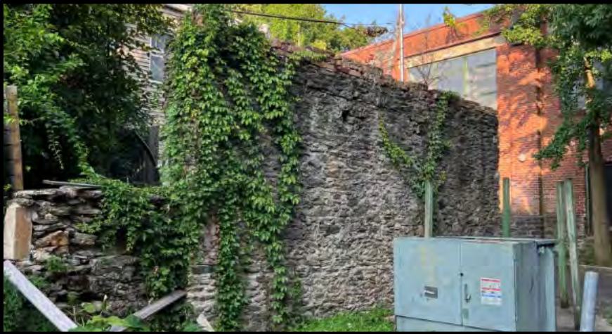
Top and middle: The NE and NW elevations. Bottom: The SW elevation of a stone wall on the subject property. Source: Keeping Society of Philadelphia, 2023.
