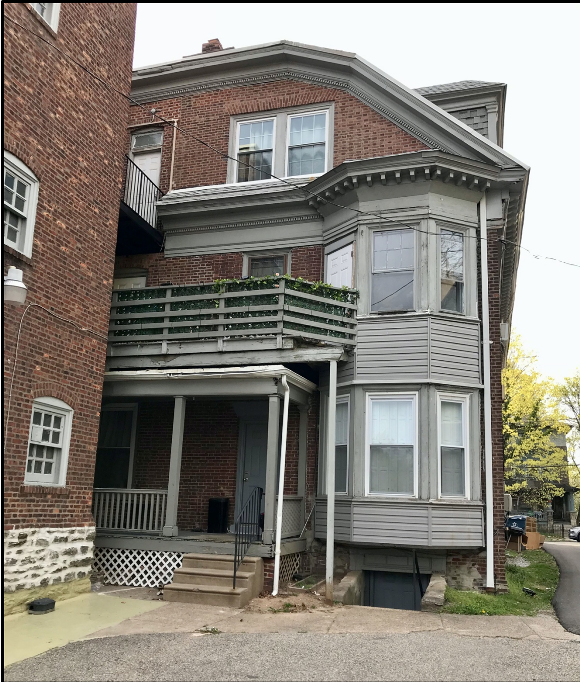
Figure 9. South elevation of the main volume illustrating original and modified elements to accommodate the current multi-family use. Source: Keeping Society of Philadelphia, 2023.
