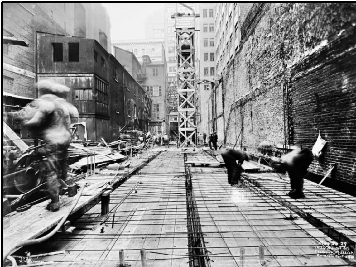
Figure 23. Looking north from the rear of the parcel at 1424 Walnut Street with Drexel & Co. in the background, employees of Frederick Massiah, a prominent African American concrete contractor, work on a new commercial building, designed for the financial industry, on May 20, 1929. Note the ubiquitous Philadelphia townhouse standing on left, which remained from Walnut Street’s residential period. Source: The Frederick and Edith L. Massiah Papers were donated to the University of Pennsylvania Archives by Louis J. Massiah in August 2011 (Accession # 2011:048).
