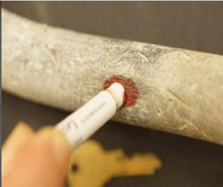
Lead Test kit– Red Dot Appears (make sure to test pipe, not paint!)
