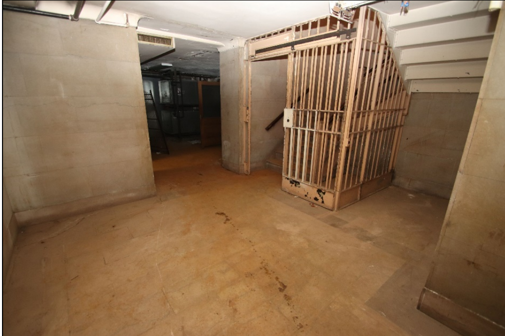
Photo 18 (left): Basement lobby, adjacent to the main stair (at center-right), looking northeast.
