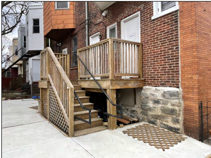
Fig. 14. North or rear elevation of both properties showing ground conditions including smoothly paved concrete where a 1923 garage once stood behind 4951.
