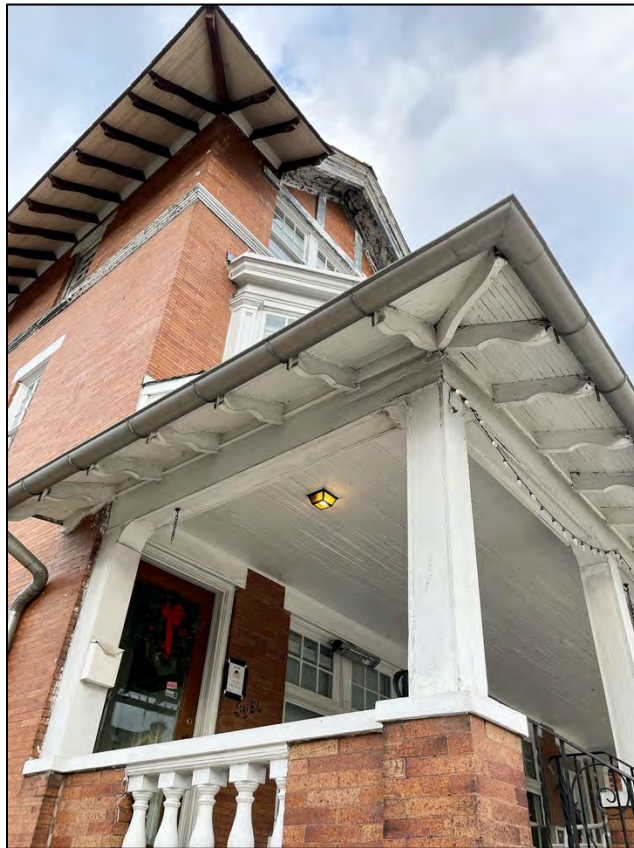
Fig. 8. Southwest corner showing the deep rafters at the porch and roof overhangs.
