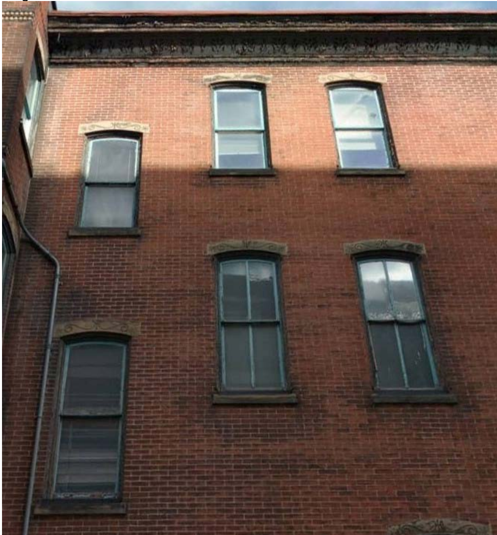
Figure 6: The southern portion of the Fitzwater Street elevation features windows with arched lintels ornamented with flourishes. Image from Cyclomedia.phila.gov
