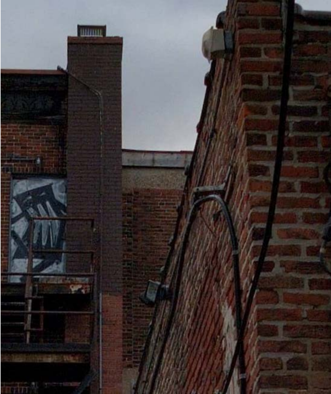
Figure 11: View of the North wall from the rear (East). 731 S. Broad Street is to the left, including the chimney.
