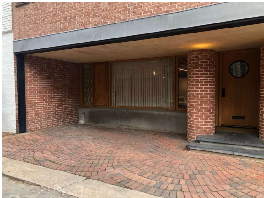
Figure 8: The recessed open space on the first floor was designed as a carport and main entrance area. The inset wall contains a picture window and two entry doors. It is not clear from research if the semi-circle paving pattern was originally installed by the architect or a later alteration.
