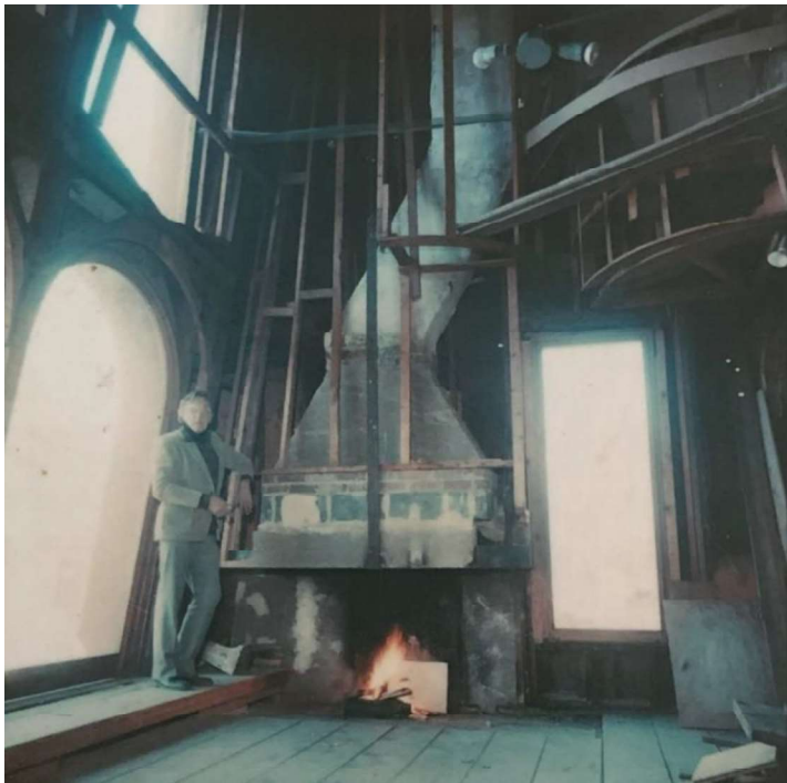
Figures 33: Interior photograph showing Frank Weise during construction on the third-floor interior. Undated photograph.
