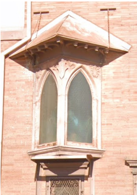
Window detail on 772, Google
