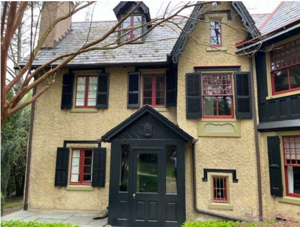
Figure 7: Detail of the South elevation, showing the enclosed entry vestibule and projecting gable. Photo by Massimo Cristofanilli.
