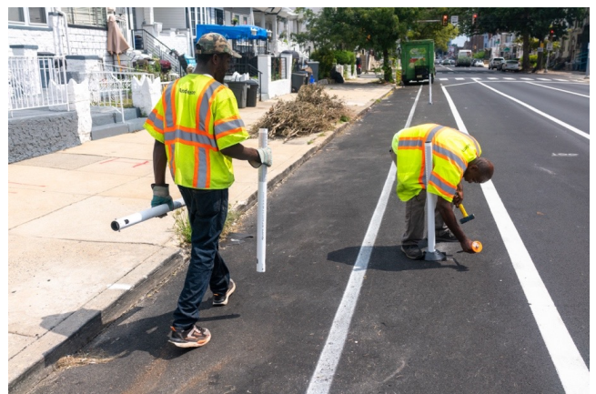
WORKERS INSTALL FLEX POSTS ON A NEWLY PAINTED PARKING SEPARATED BIKE LANE ON CHESTNUT STREET NEAR 57TH STREET.
