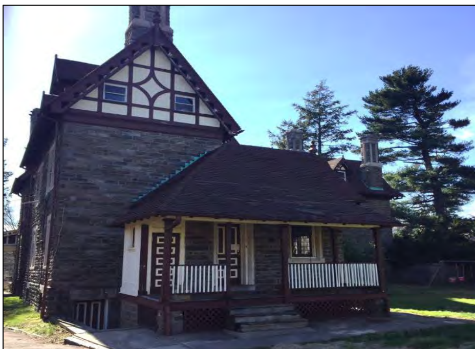
Photo 10. Northeast (rear) elevation showing the one-story room and porch with small enclosure, facing west.
