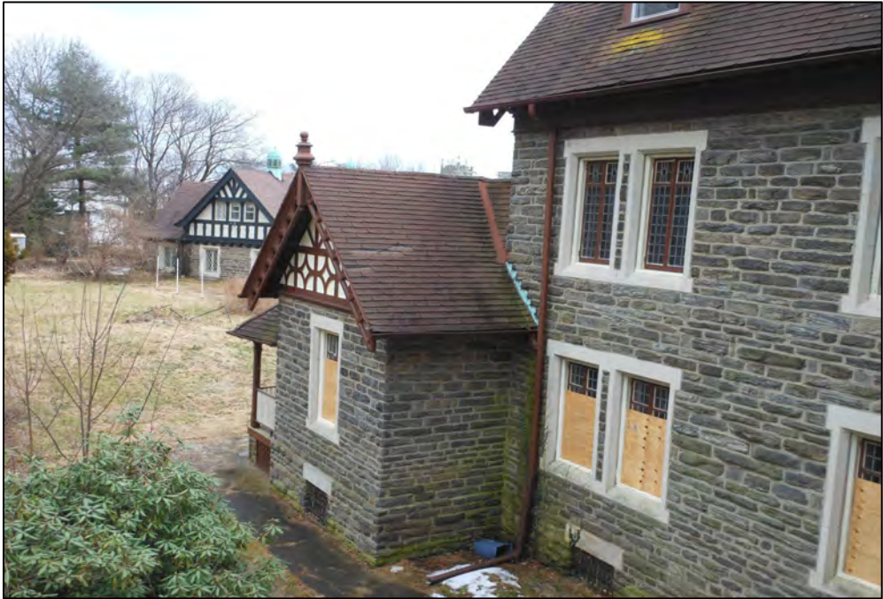
Photo 30. Carriage house as seen from the main block of the house, facing east.
