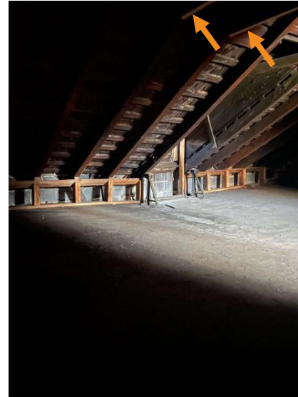
Figure 4. Photo included in application, with arrows added to show existing collar ties at No. 212
