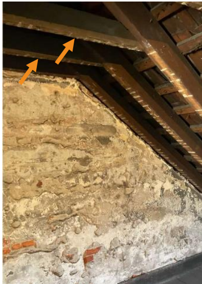
Figure 3. Photo included in application, with arrows added to show existing collar ties at No. 208
