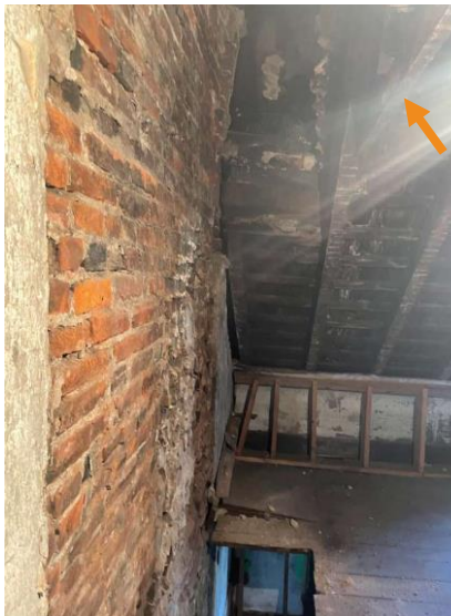
Figure 2. Photo included in application, with arrow added to show existing collar tie at No. 208
