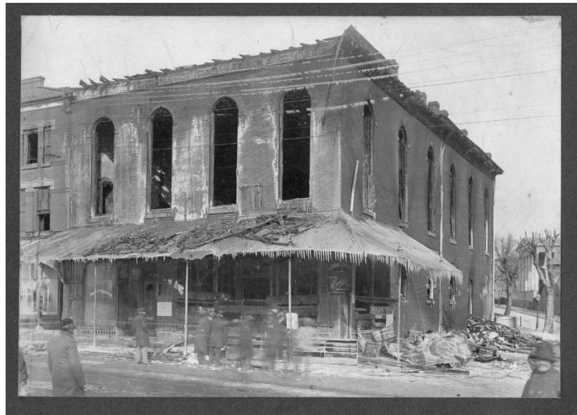
Figure 21: Parker's Hall after a fire that gutted the building, ultimately leading to its demolition and the reconstruction of a new building on the remaining foundation (the building which stands today.) "Parker Hall fire," erroneously dated 1899. Germantown Historical Society. https://germantownhistory.catalogaccess.com/photos/8815 .
