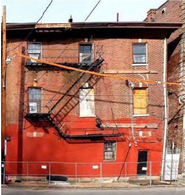
Figure 9: A 2017 photograph of the eastern side of the southeast elevation features the dramatic bend of the structure's east corner that demanded structural remedy, seen below. The foundation may date to the 1870s and is presumed to be a contributing factor to the structural instability. (Photo by Sara Stratte.)
