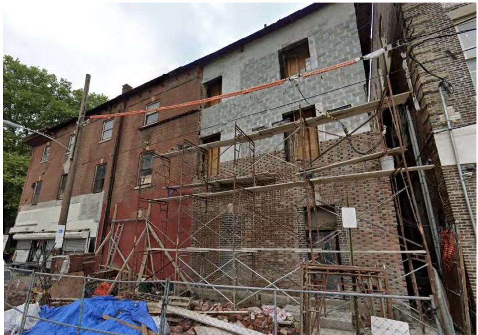
Figure 10: This photo from Google Streetview shows the stabilization and reconstruction efforts underway in 2019. The rebuilt portion uses concrete masonry units clad in brick.
