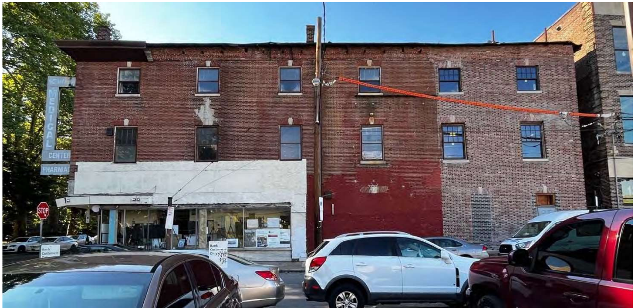
Figure 8: Price Street (Southeast) elevation of 5801-03 Germantown Ave. Photo by Nika Faulkner. Note the new matching windows, Flemish bond brick veneer that differs in color, and lack of cornice.
