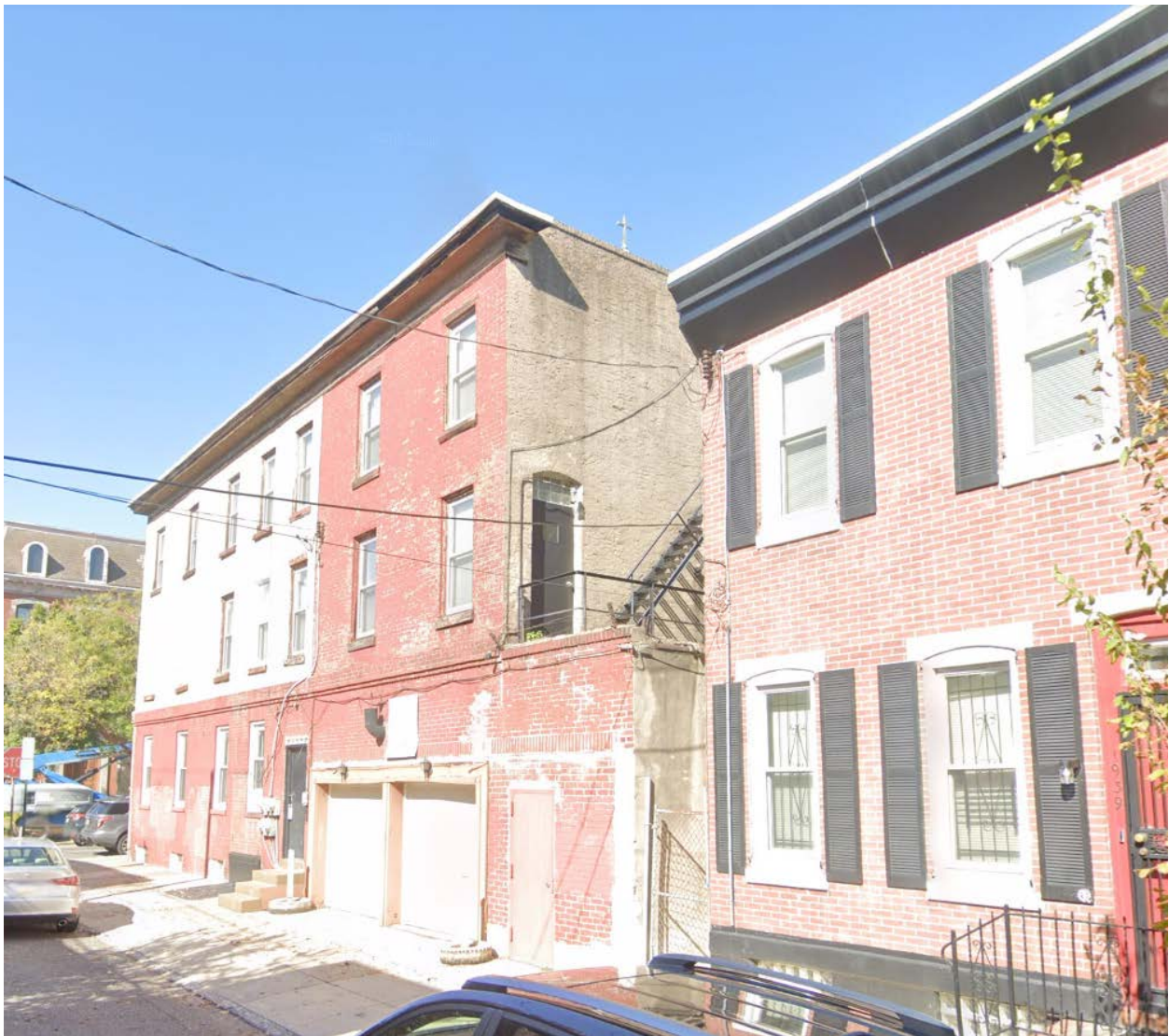
Figure 5, view of the easternmost final bay on the southern façade including fire escape and exit, added later.
