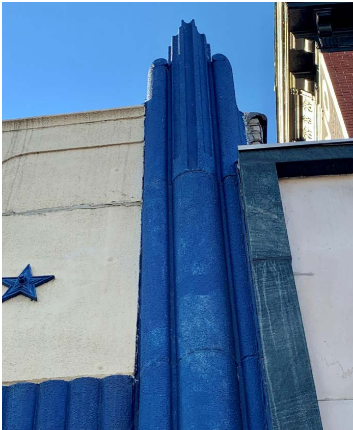
Figure 8. Close-up view of piers and texture of painted concrete "cast stone" panels, December 2022.
