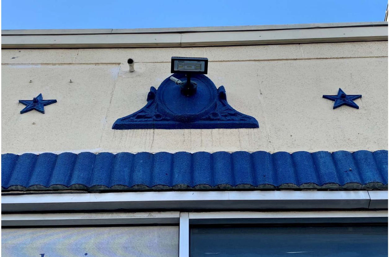
Figure 3. Medallion ornamentation with modern light fixture installed, above storefront windows on South Broad Street elevation, December 2022.
