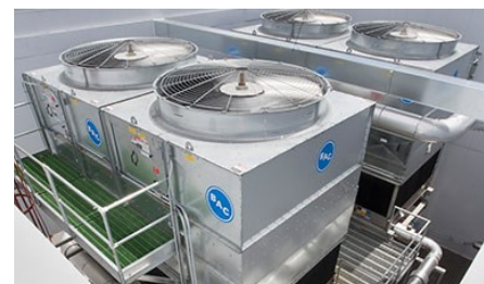
Figure 2. Building Cooling Tower
