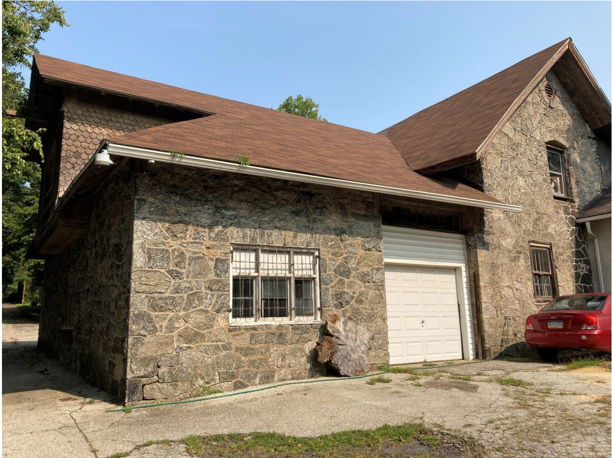
Figure 17: September 2022 photograph showing current conditions of the carriage house. View looking northeast.
