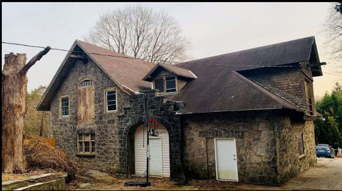
Figure 67. Top: Looking south at the Carriage House & Stable. Source: Pictometry, Atlas, City of Philadelphia. Figure 68. Bottom: The primary (northwest) elevation of the Carriage House component of the larger Carriage House & Stable. Source: Oscar Beisert, 2019.
