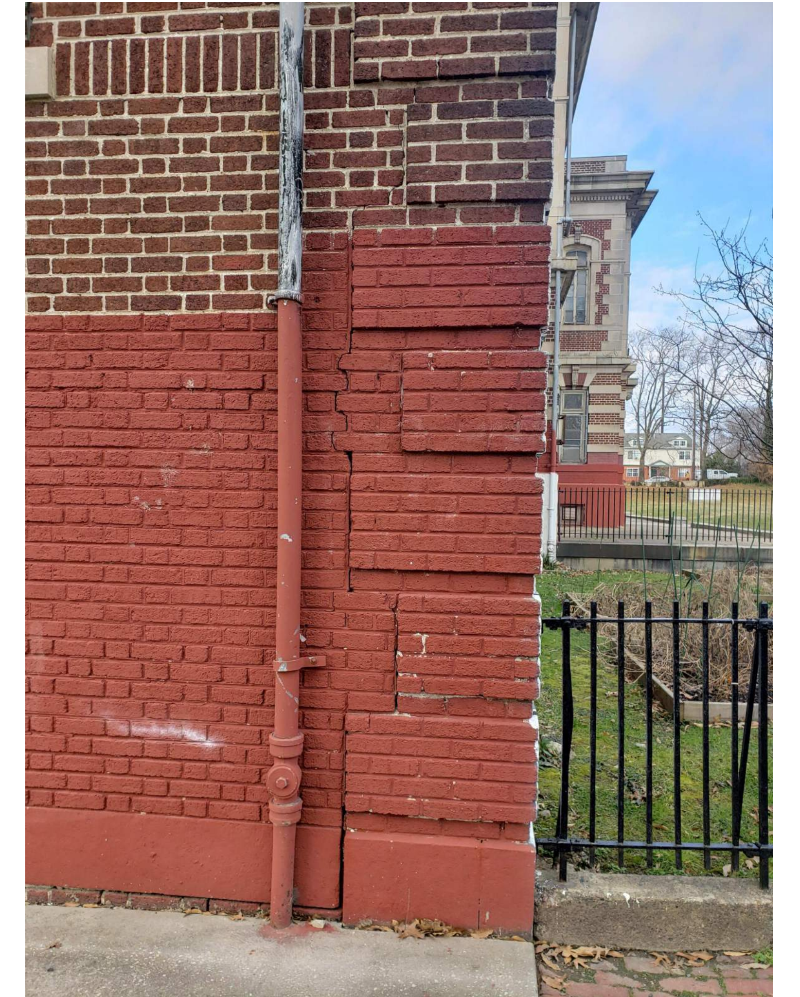
MASONRY CRACKS - SOUTH ELEVATION
