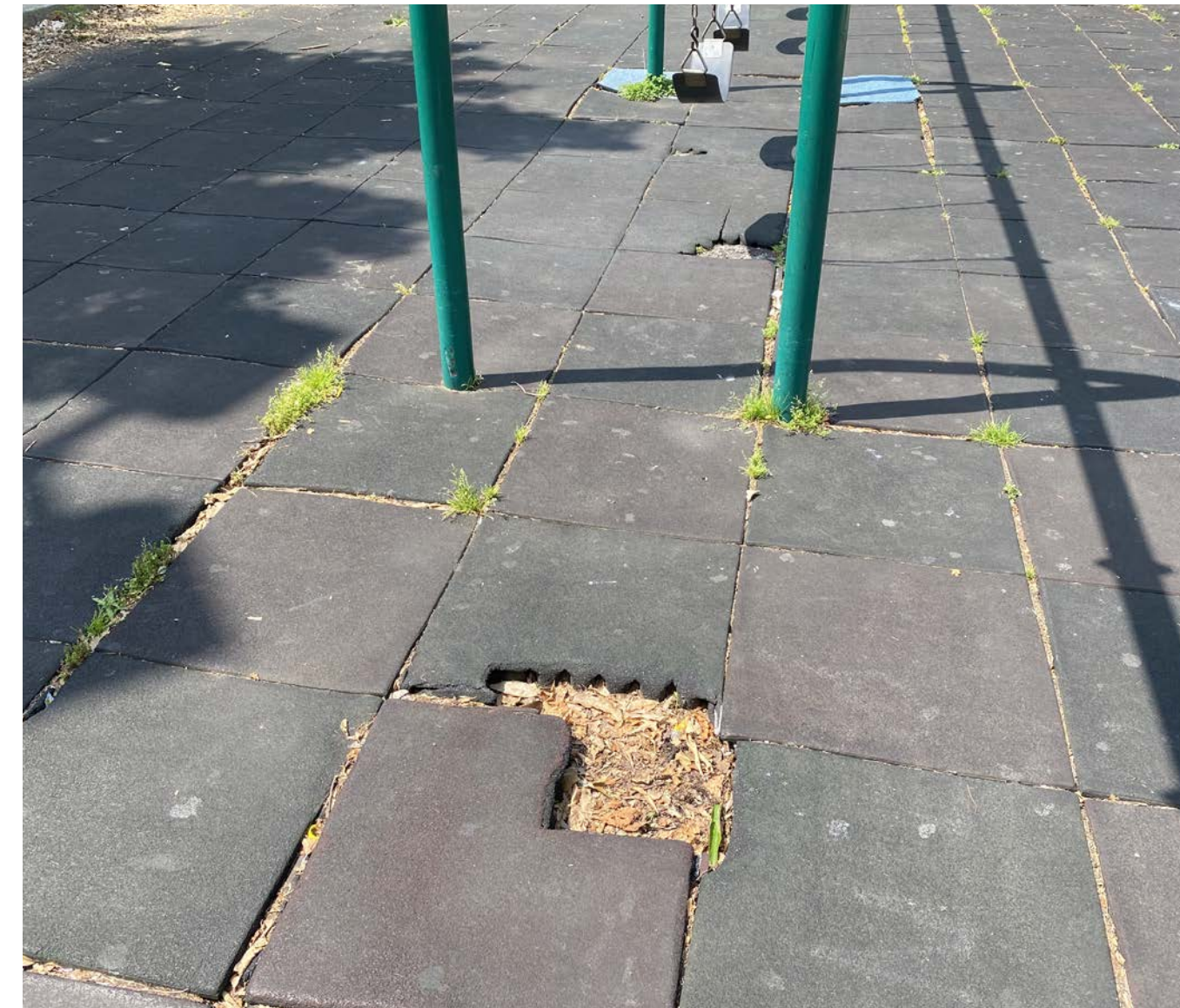
2 DAMAGED PLAYGROUND SURFACING
