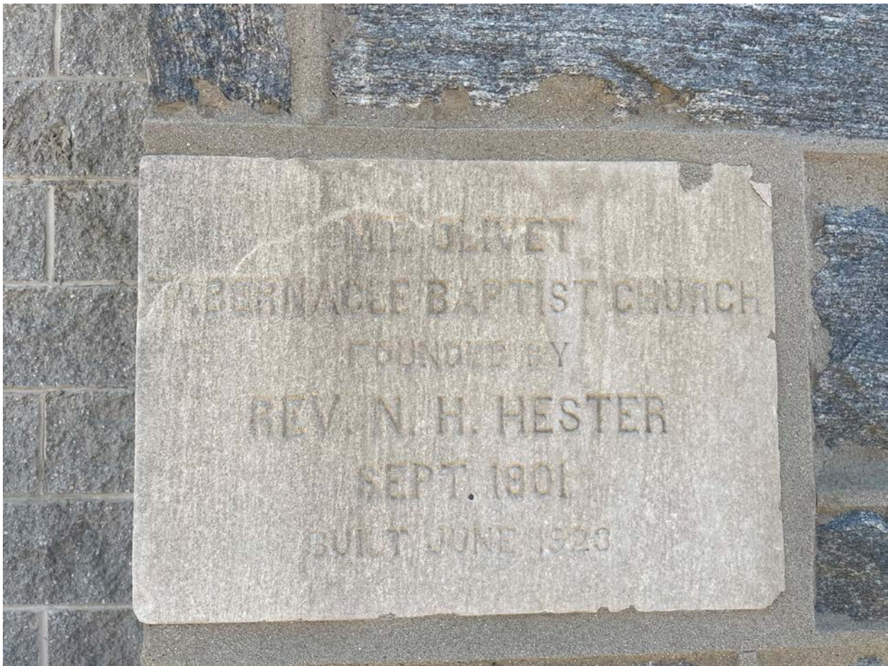
Figure 14. Detail, west facade, Mount Olivet Tabernacle Baptist Church. Photo: Corey Loftus, July 2022.
