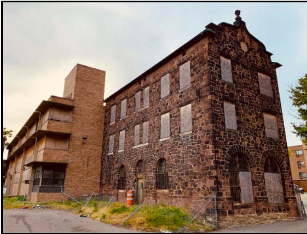
Figure 1. The east and south elevations of the Infirmary and Infirmary Addition. Source: Oscar Beisert, 2021.
