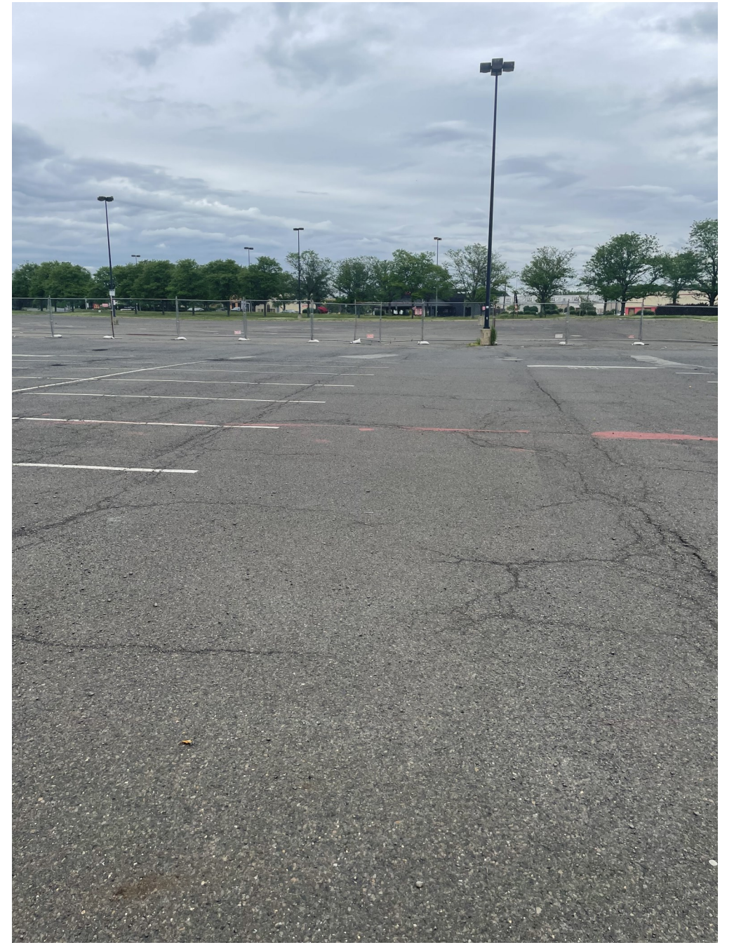
Photograph 3 - View looking northeast at the location of the proposed parking lot improvements into the site.
