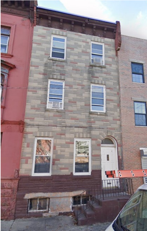
Example of 1.b.ii: The PermaStone veneer at 1842 Christian Street has been attached to the original façade rather than replacing it; the older façade remains underneath.
